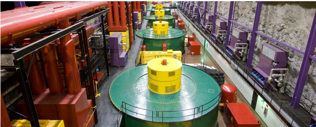
Figure 17-3 — Typical Hydroelectric Power Turbine Hall
