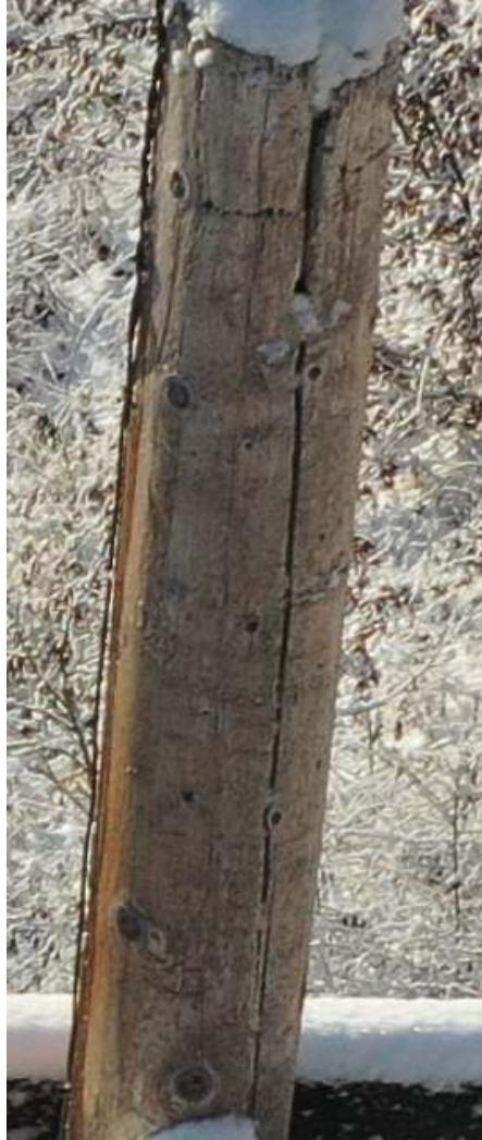
Structure K426-11: - Upper Pole Splitting
