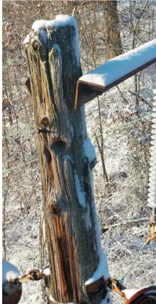
Structure K426-12: - Upper Pole Decay - Pole Cavities
