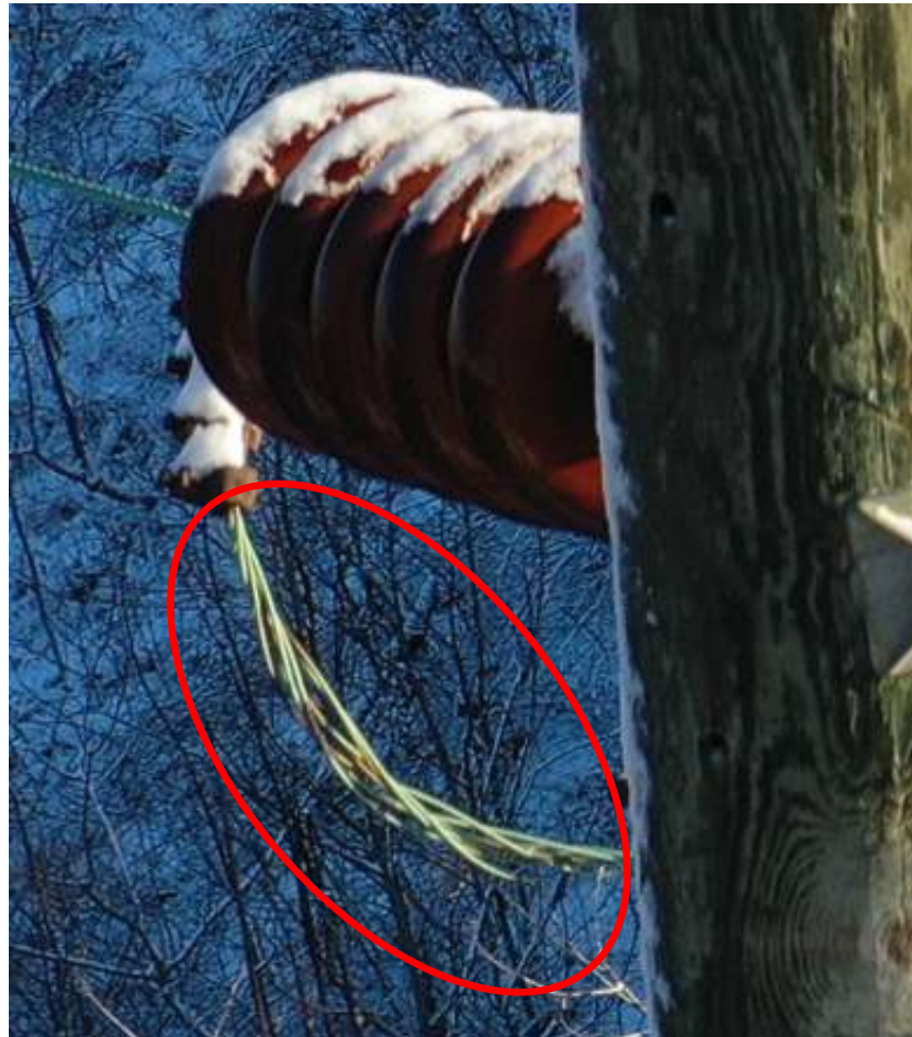
Structure K426-12: - Conductor Jumper Uncoiling - Evidence of Arcing
