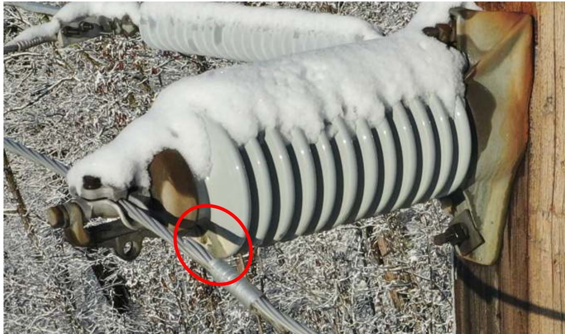
Structure K426-36: - Minor Insulator Flashover Evidence
