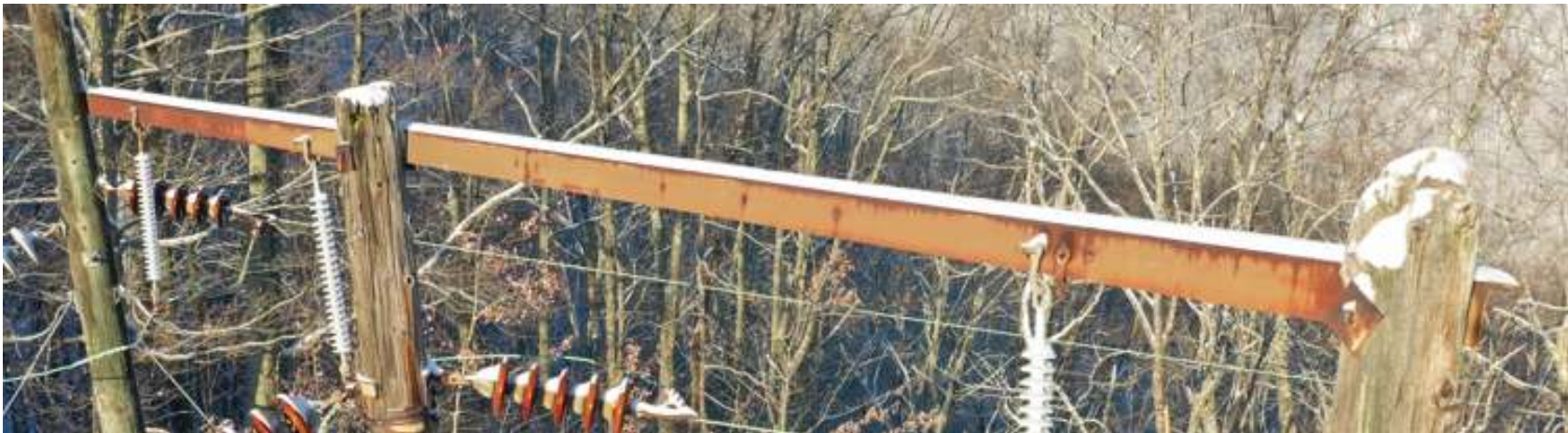
Structure K426-12: - Crossarm and Hardware Rusting
