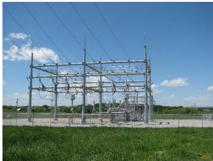
Figure 1: Comparable Proposed Substation
