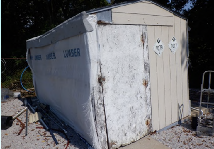
Before: Failing disinfection shed, no safety rails around treatment basin
