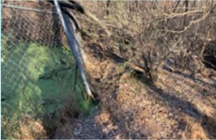
Before: Rusted tank, compromised fencing
