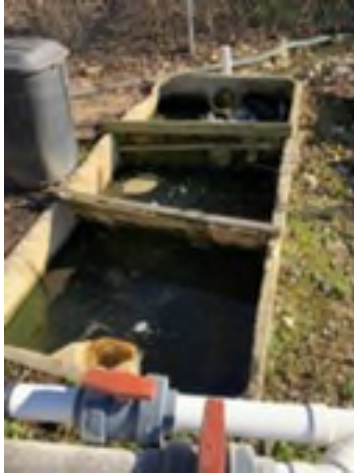
Before: Clogged contact chamber, channel erosion
