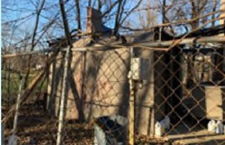
Before: Deteriorated service area, no safety rails
