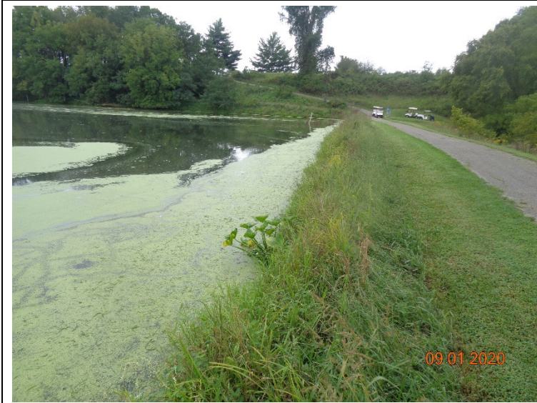
UPSTREAM SLOPE – LEFT VIEW GRASS NEEDS TO BE MOWED
