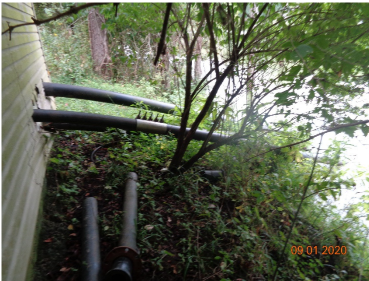
PUMP HOUSE - ALONG BANK BELOW UPSTREAM DAM USED TO DRAW DOWN LAKE FOR IRRIGATION
