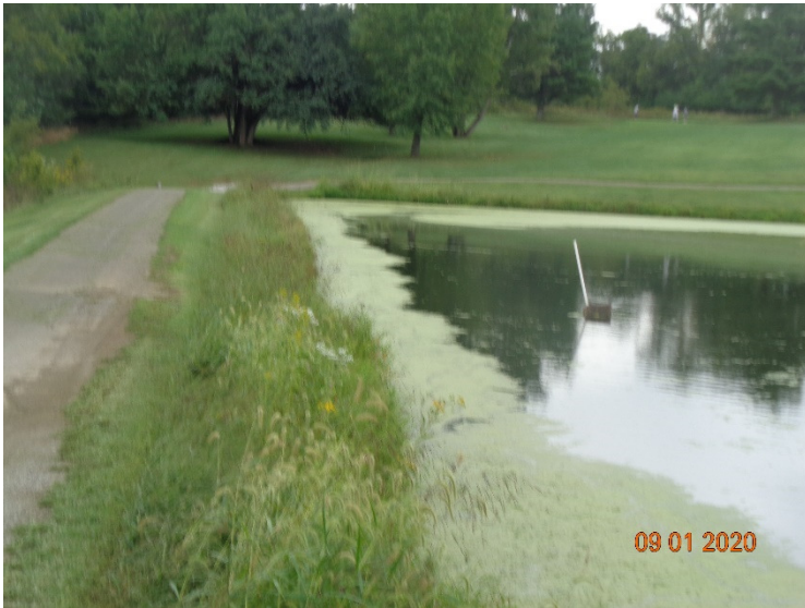
UPSTREAM SLOPE – RIGHT VIEW GRASS NEEDS TO BE MOWED
