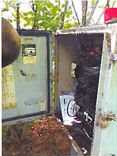
Lift station control panels appear to be poorly wired and are a safety concern.
