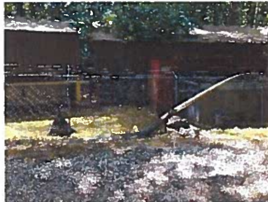
Influent PVC line is fastened to the top of the fence and should be properly buried.
