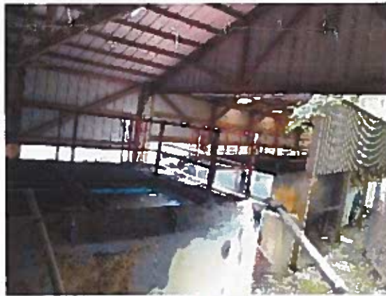
Treatment Tanks are rusting and have gone unmaintained
