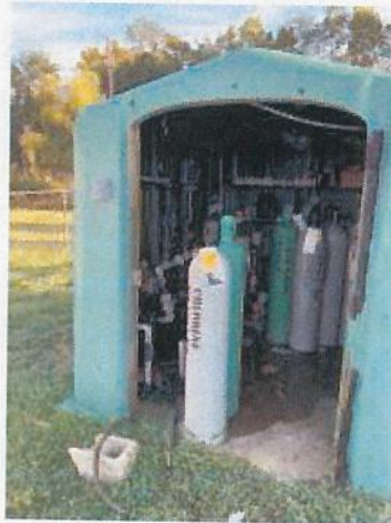
Gaseous Chlorine Storage
