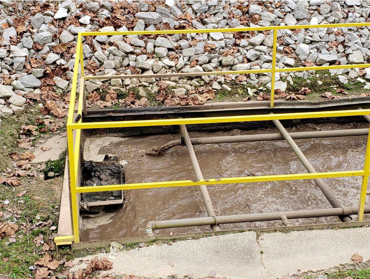
Influent bar screen, aeration, and return sludge.
