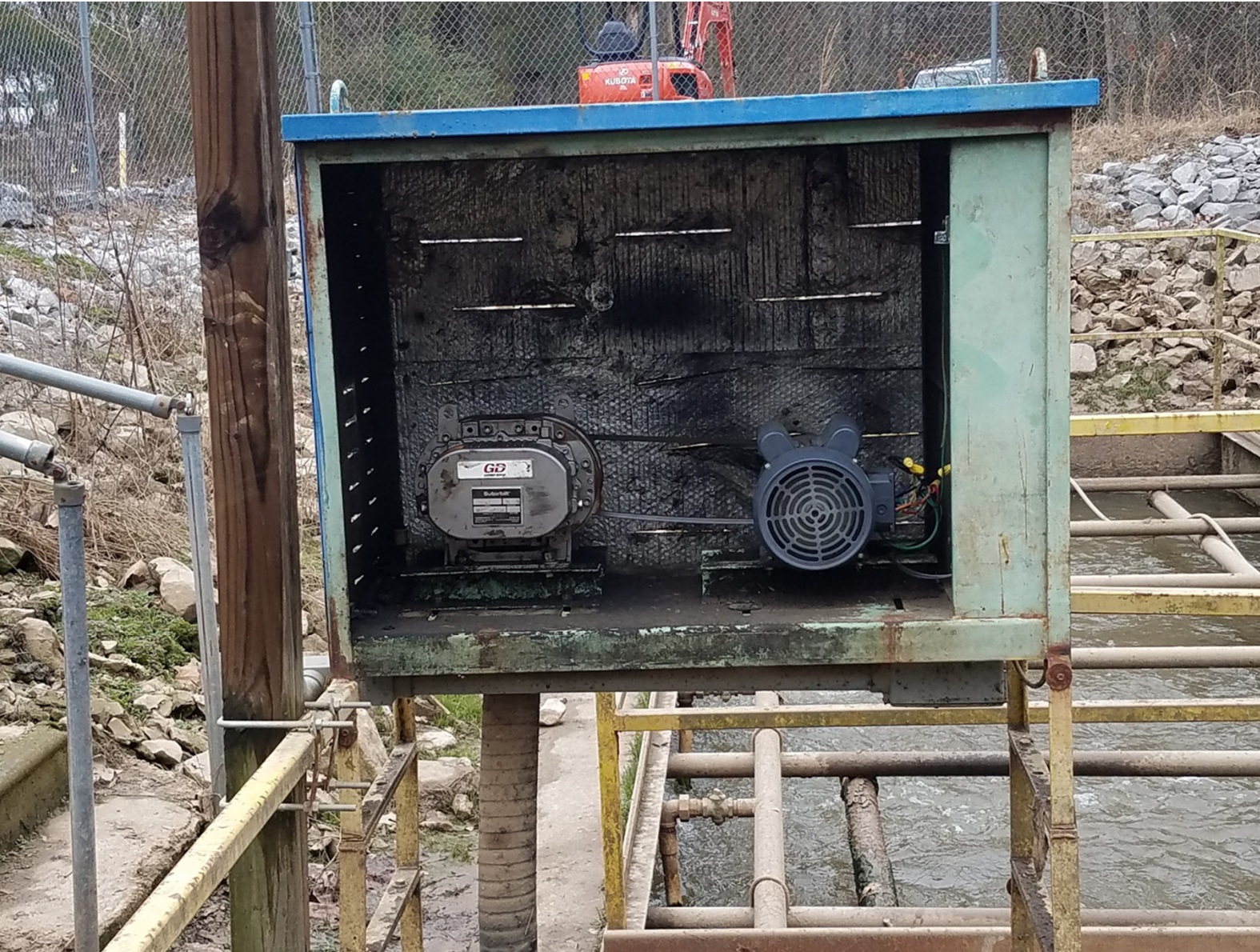
New motor for aeration pump.
