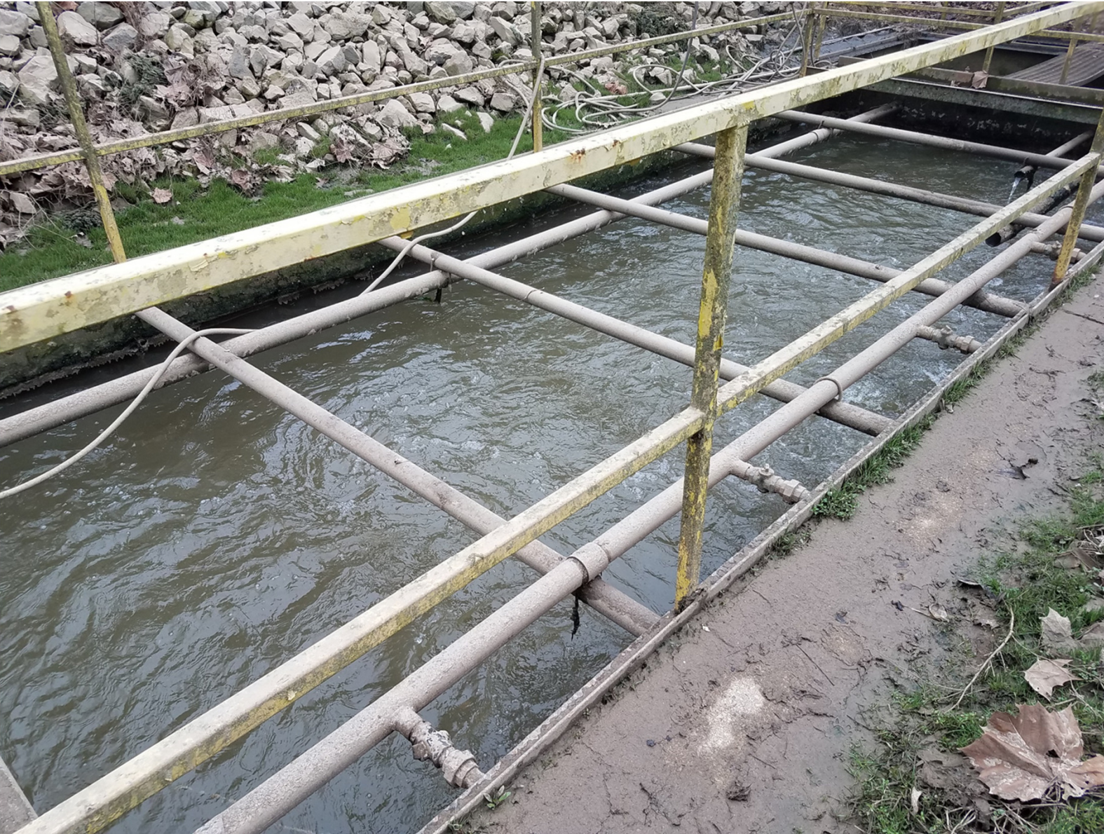
Aeration chamber. Good mixing. Low MLSS concentration.
