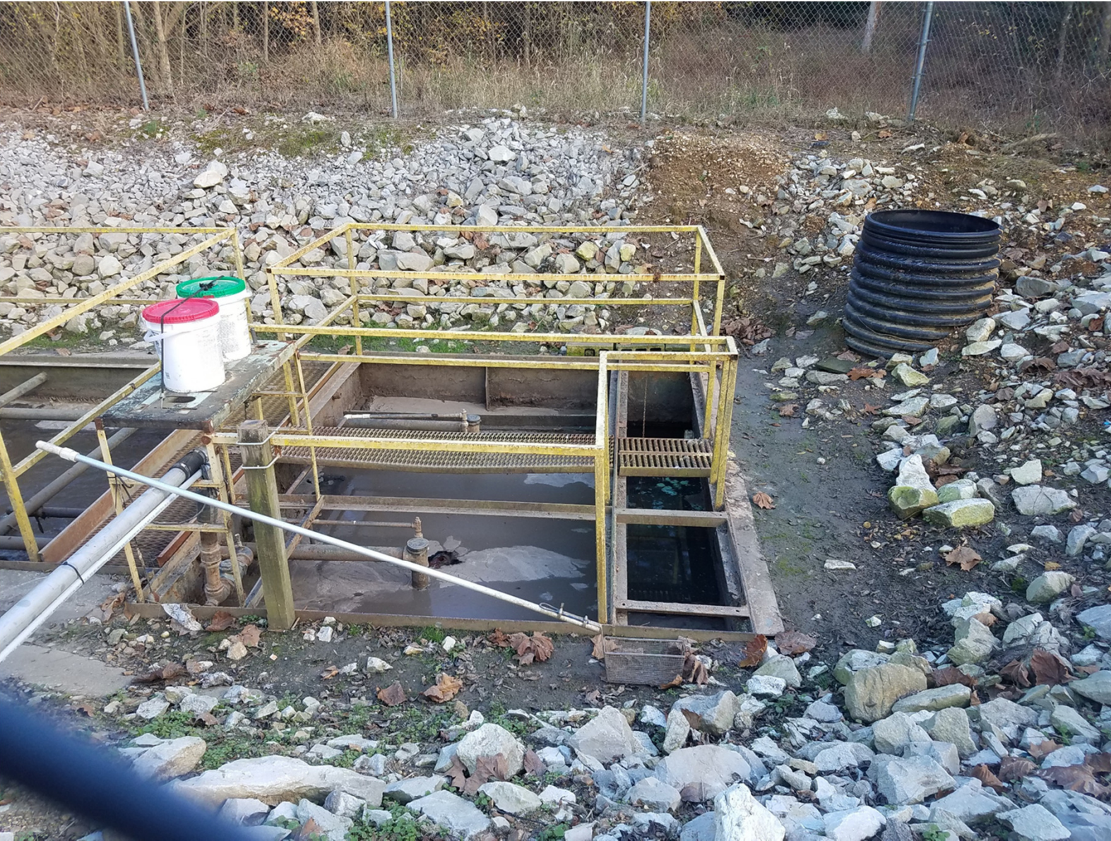
Clarifier and contact chamber
