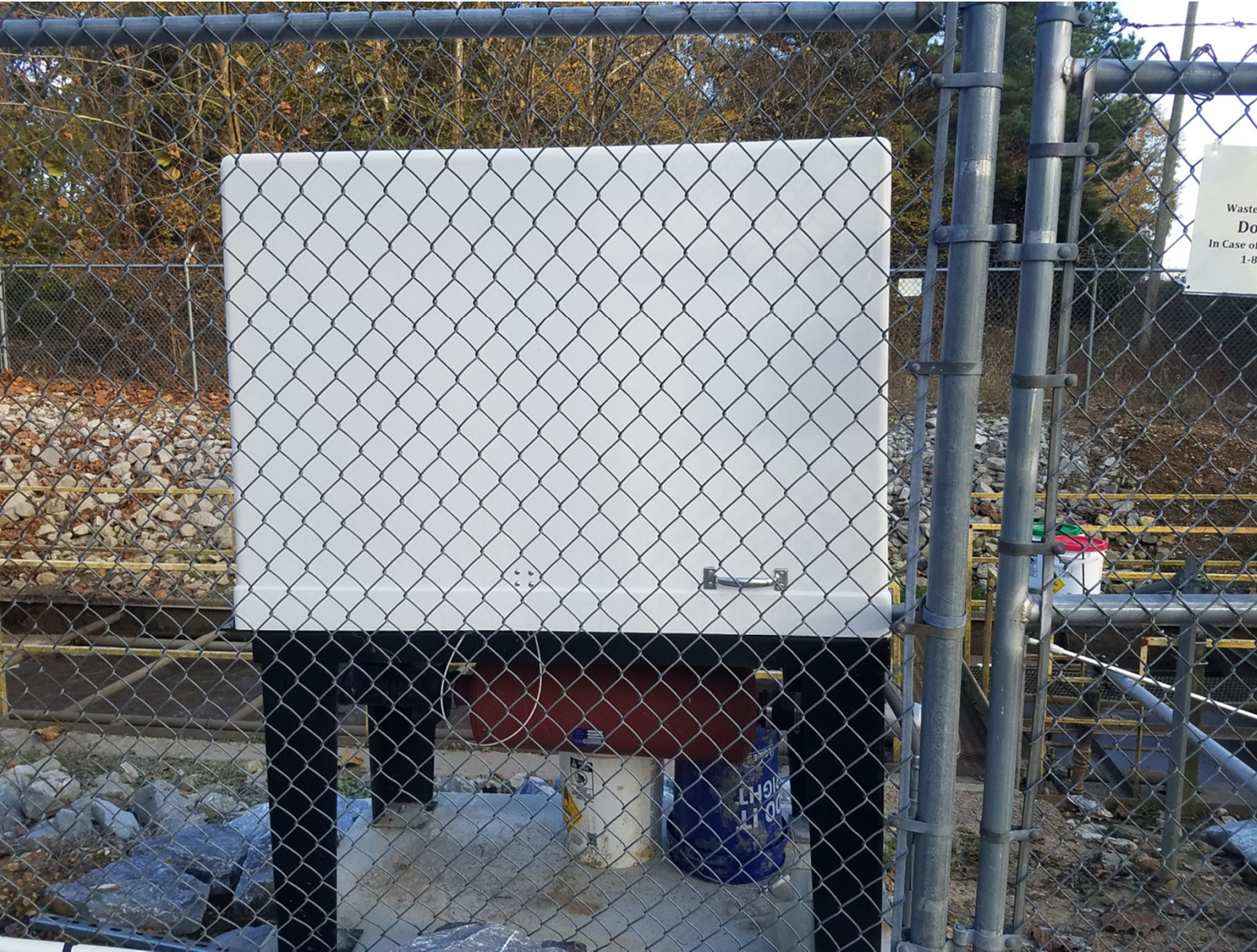
New blower motor
