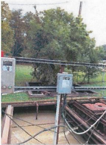
Electrical Boxes and Electrical Cabling
