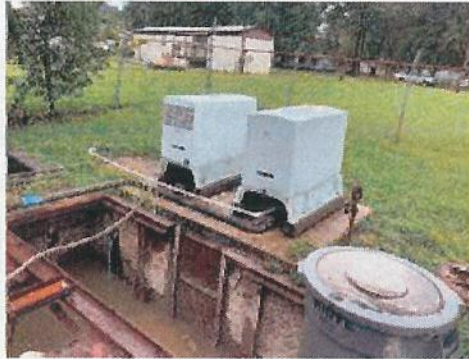
Blowers, EQ Basin, and Electrical Cables
