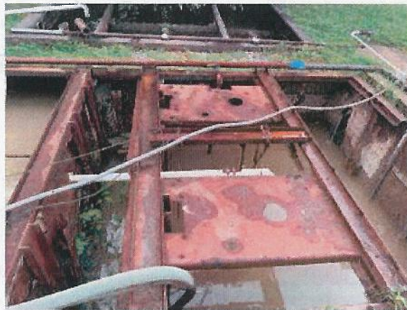
EQ Basin, Portable Pump Discharge, Digester, Miscellaneous Electrical Cables
