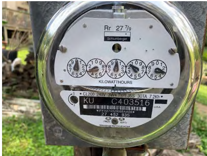
WWTP Electrical Meter
