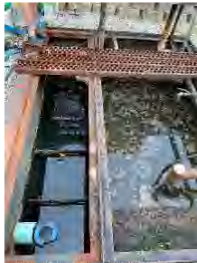
Clarifier and Contact Tank
