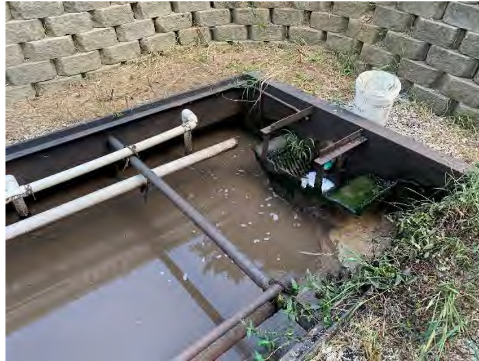
Manually Cleaned Bar Screen
