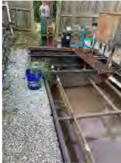
Aeration Tank, Clarifier, Contact Tank
