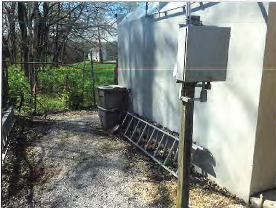
Fenced needs repaired
