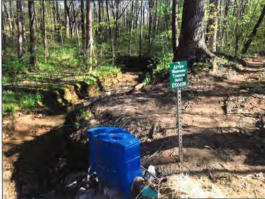
Effluent discharge point with de-chlorination unit and KPDES sign
