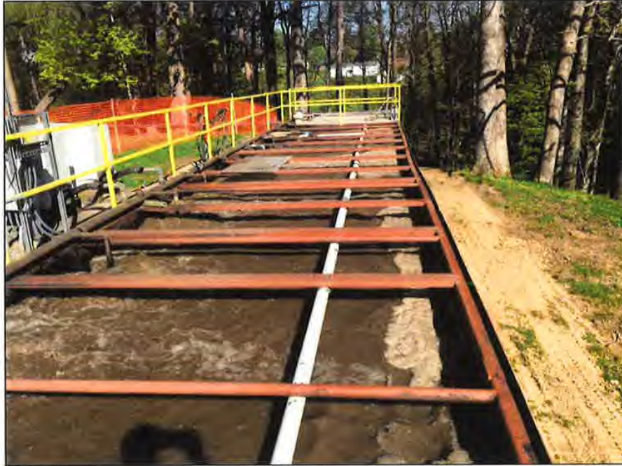
Mixed liquor in aeration basin
