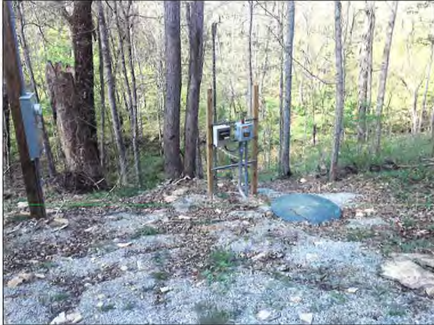
New lift station with a monitoring system
