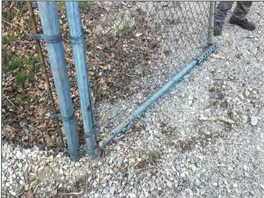
Entrance gate needs repaired
