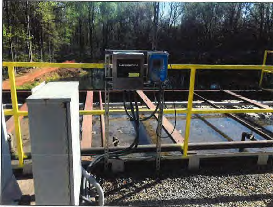
Mission-Manage SCADA Control monitoring system
