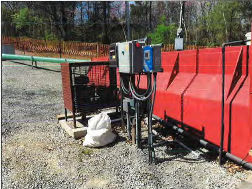
Monitoring System and Blower/motor unit
