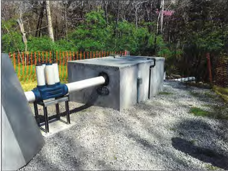
New Chlorine Contact Basin
