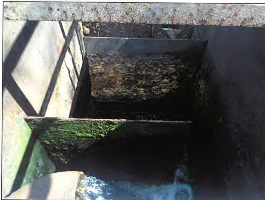
Old chlorine contact basin showing signs rust and deterioration
