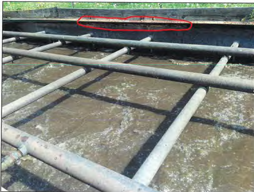
Aeration Basin – Signs of deterioration
