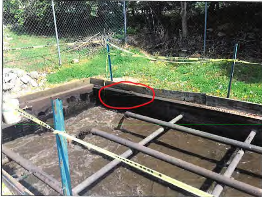
Aeration Basin – Metal Degradation
