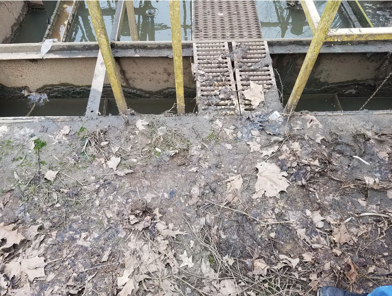
Solids on the ground
