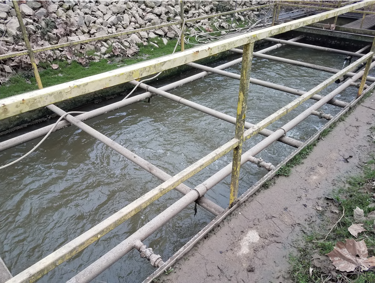
Aeration chamber. Good mixing. Low MLSS concentration.
