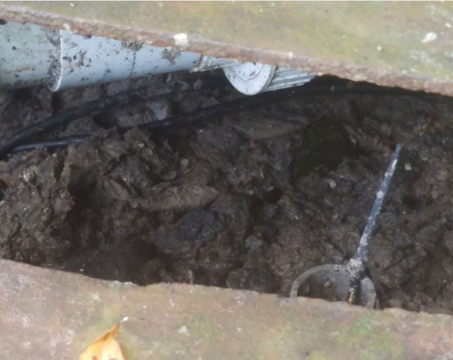
Lift station full of solids
