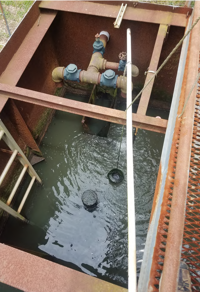
Post aeration and de-cl2 chamber
