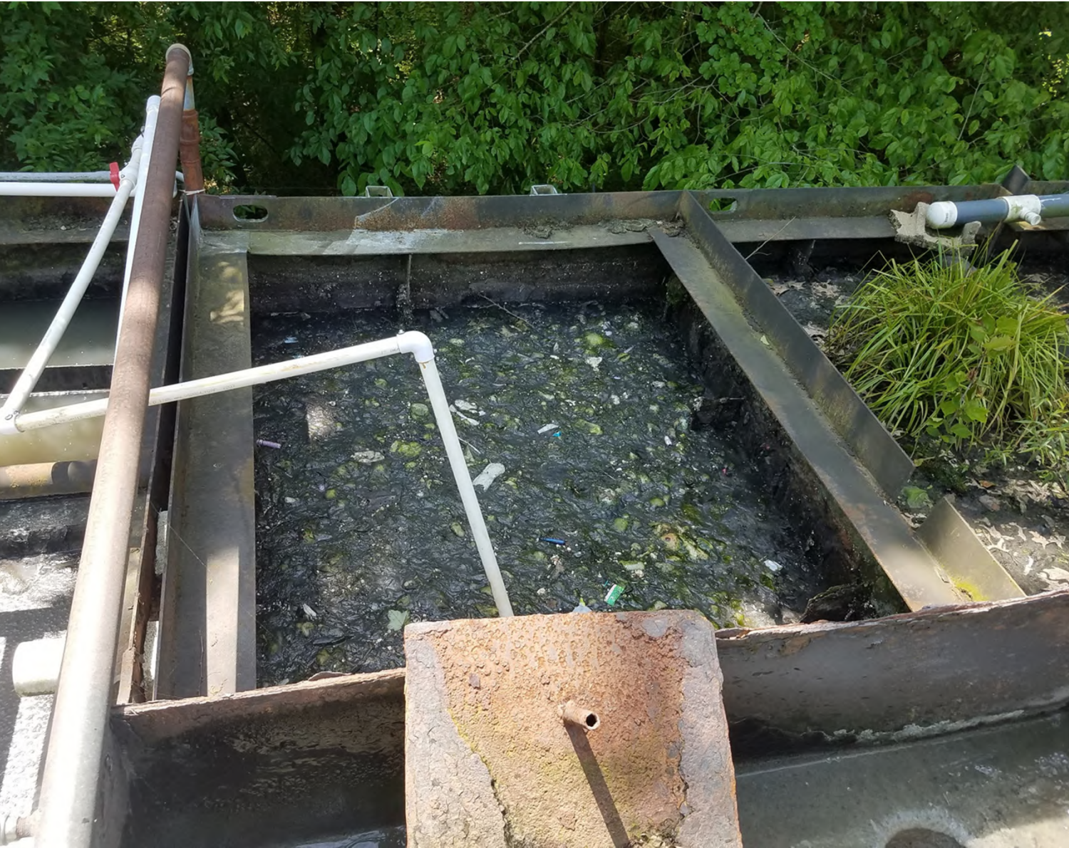
Solids in the aerator
