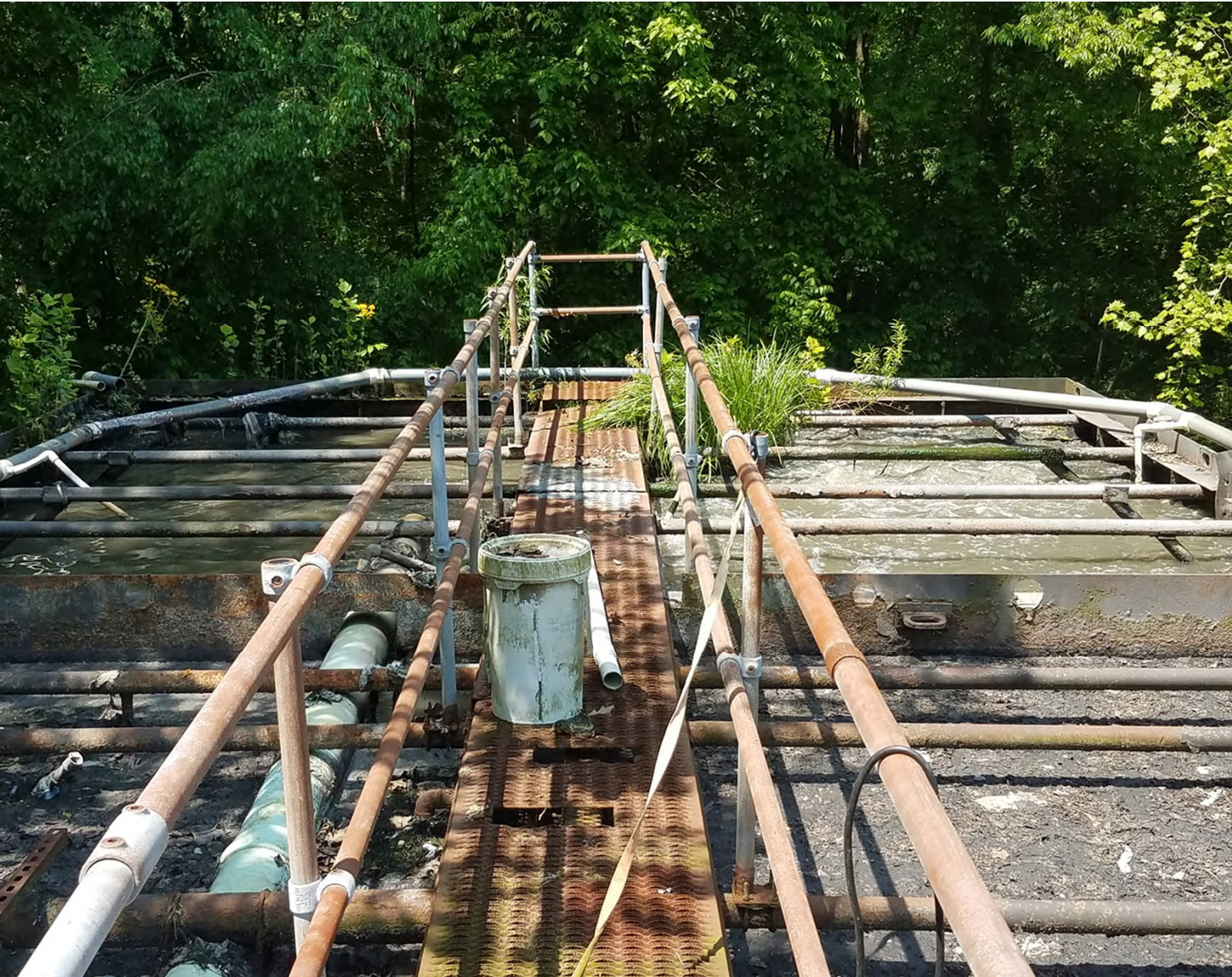
Solids in the aerator
