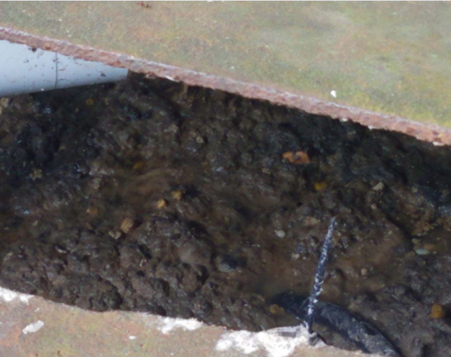
Failed lift station full of solids
