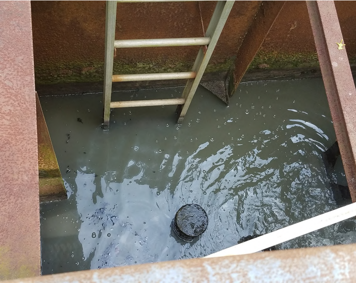
Post aeration and de-cl 2 chamber
