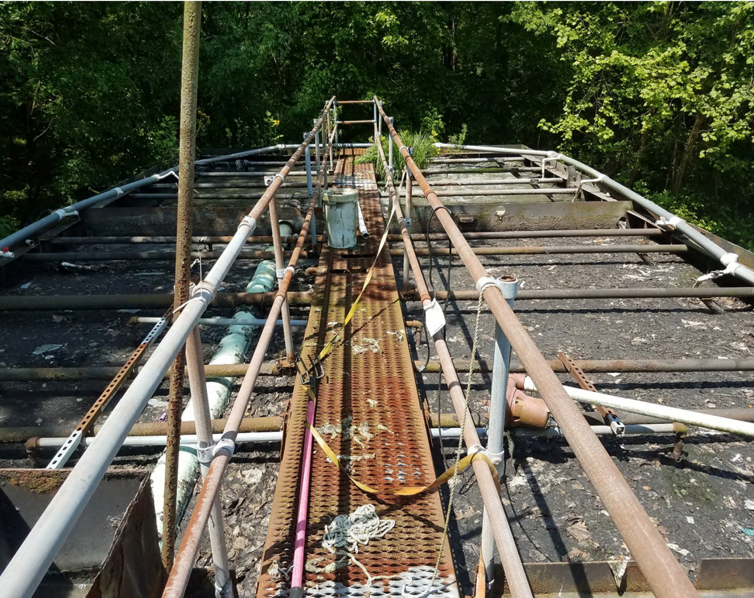
Solids in the aerator
