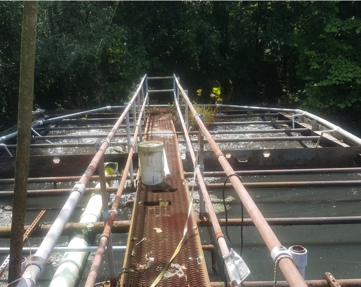
Trees growing in the aeration chamber
