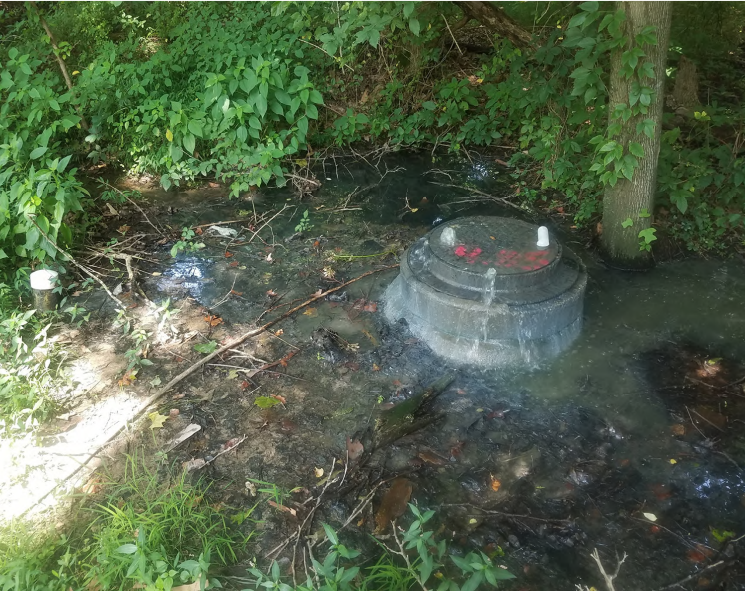
Manhole at 5730 Majestic Oak Drive overflowing.
