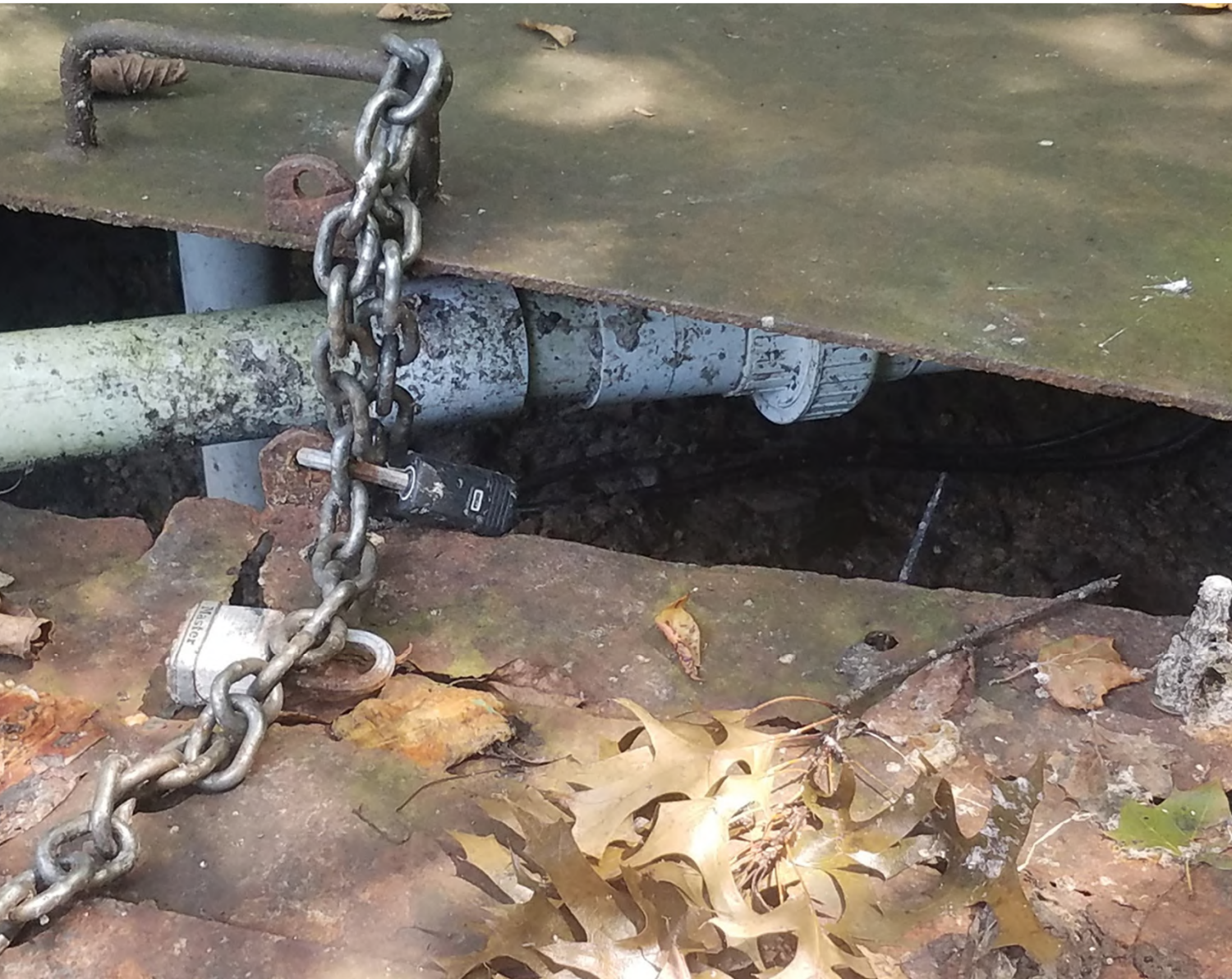
Lift station full of solids
