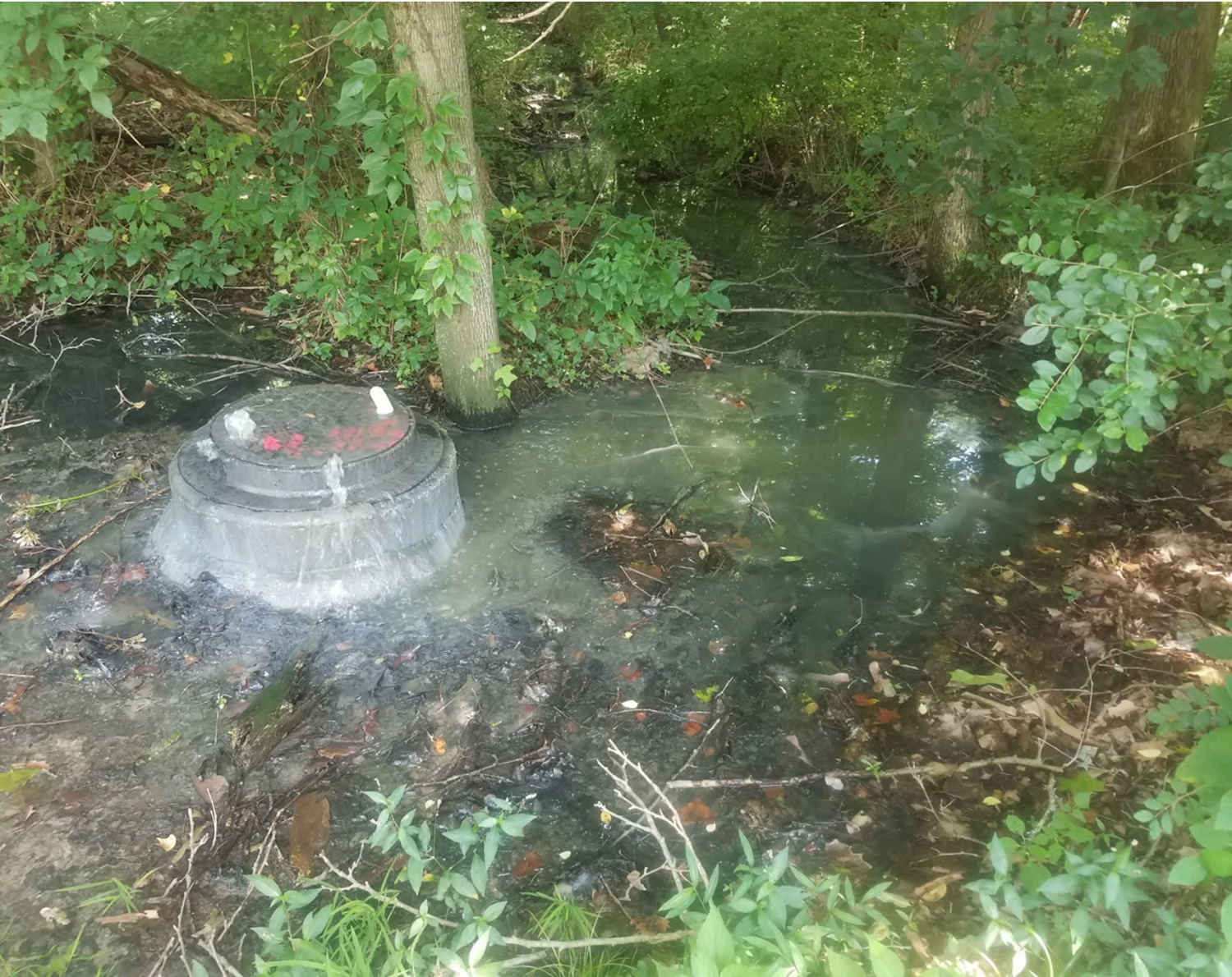
Manhole at 5730 Majestic Oak Drive overflowing.
