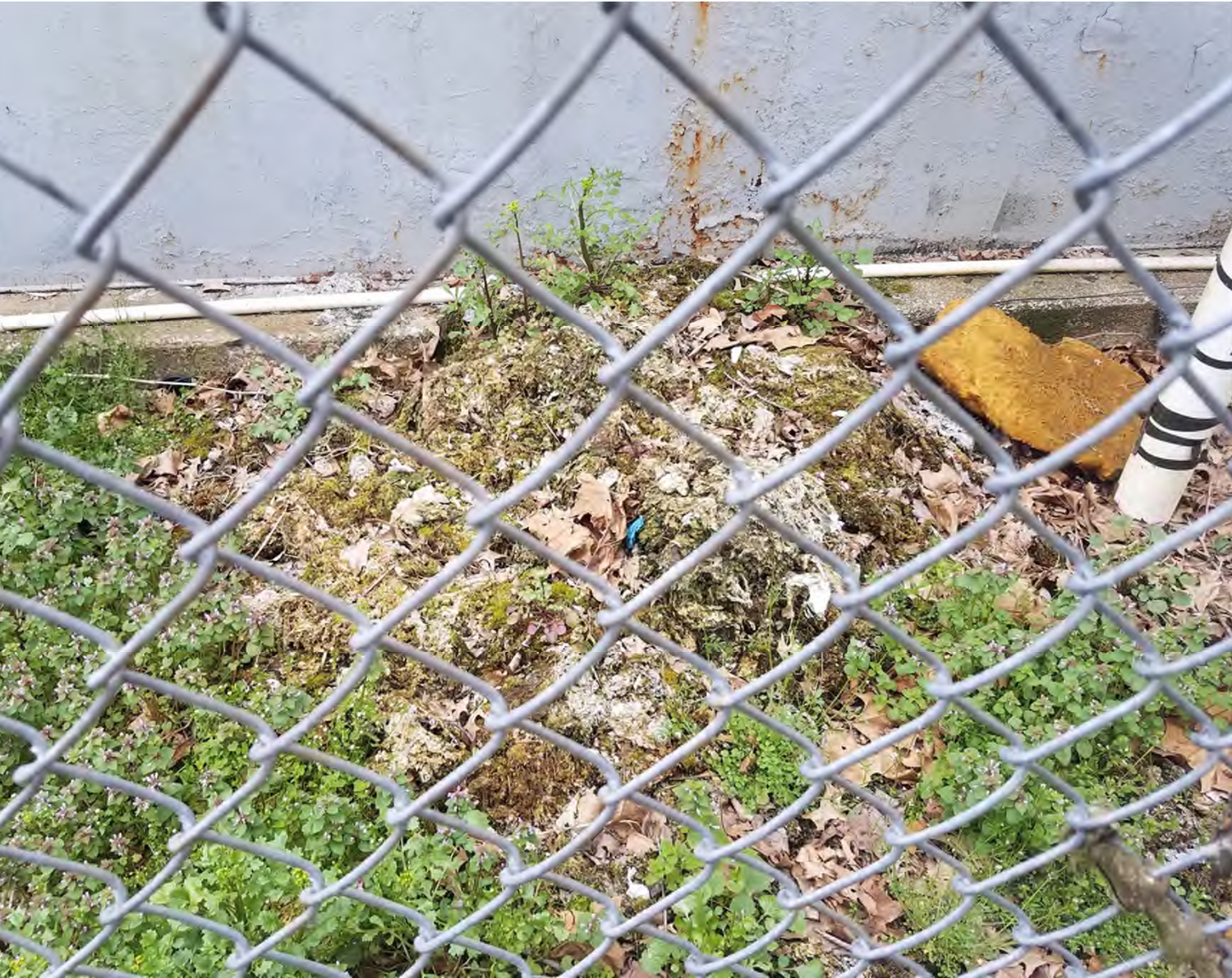
Solids on the ground beside the plant.
