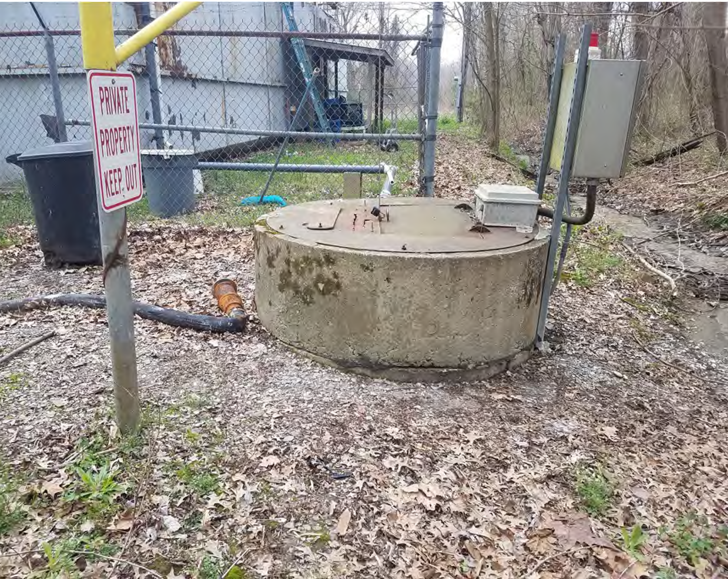
Influent lift station.
