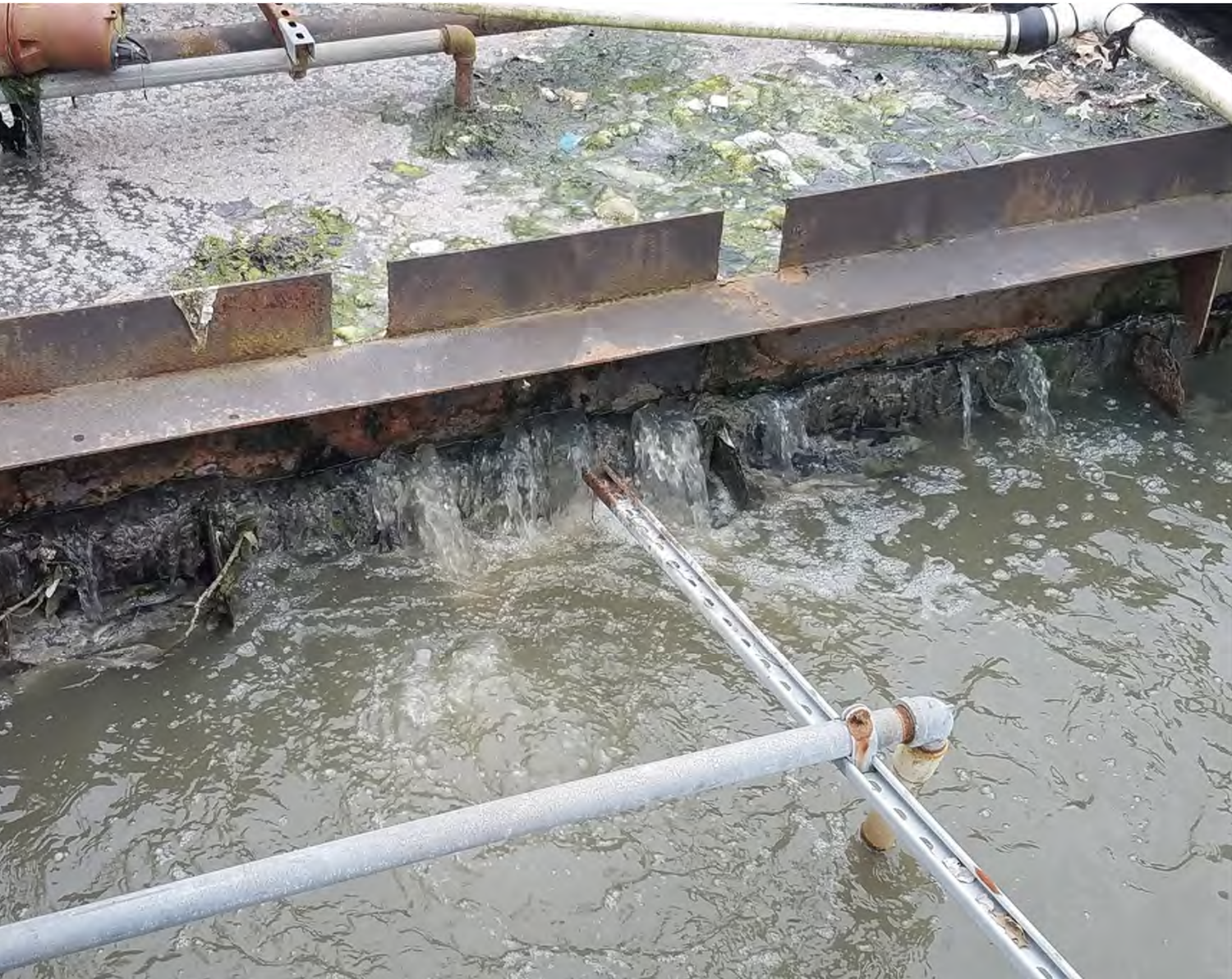
Aerator spilling over into the clarifier
