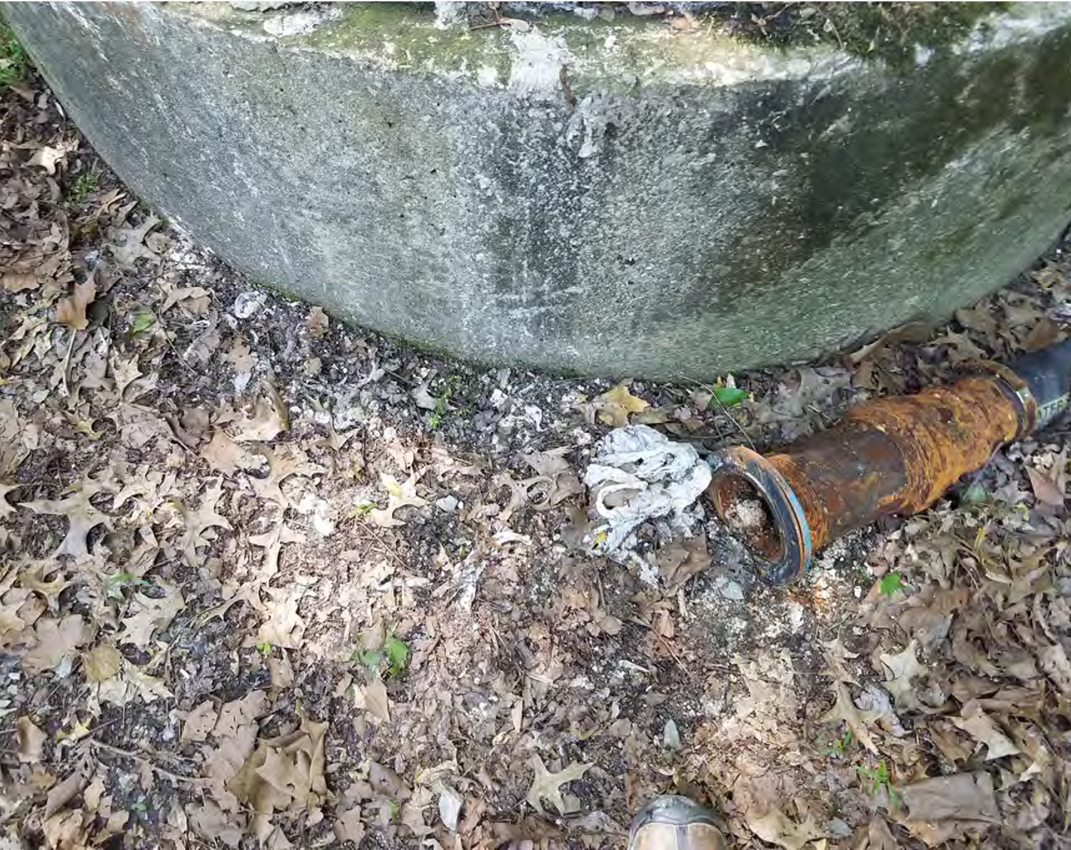
Solids on and near the lift station
