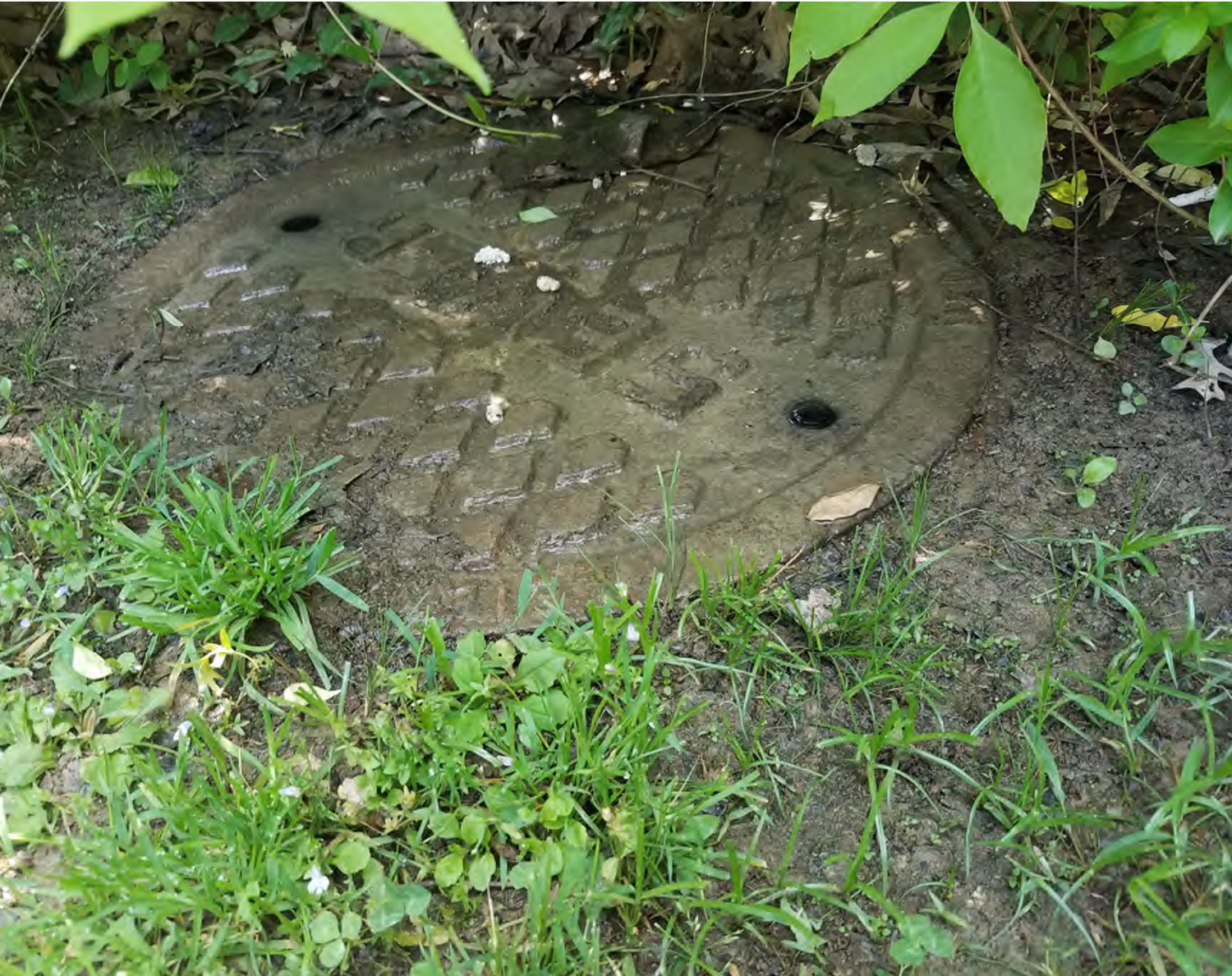
Overflowing manhole at 5700 Majestic Oak Drive
