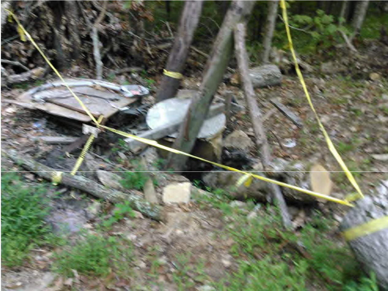
Fox Run WWTP, Frankfort, KY September 17, 2015. Deborah Singleton, Environmental Inspector. Lift station hit by trees in July 2015.
