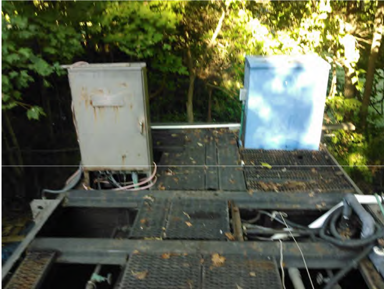
Fox Run WWTP, Frankfort, KY September 17, 2015. Deborah Singleton, Environmental Inspector. View toward chlorine contact basin.
