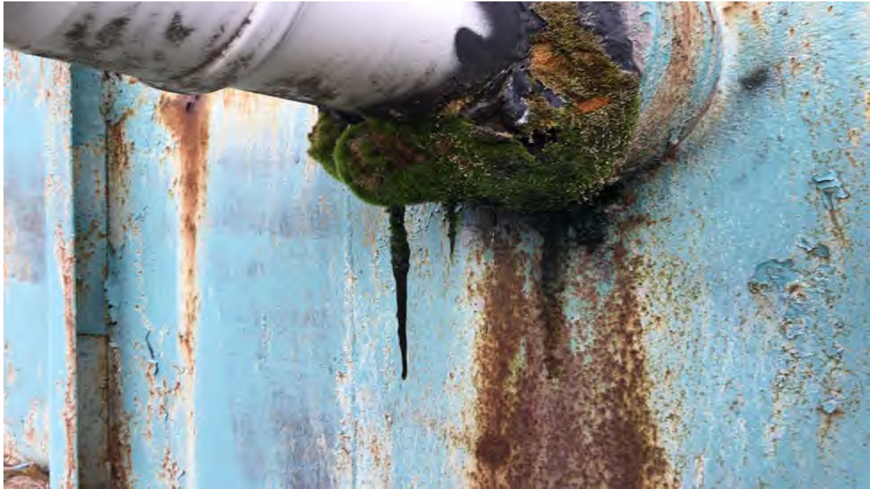
Closer view of leak
