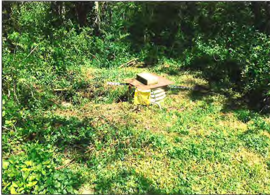
Mitchell Drive Lift Station - Before Replacement
