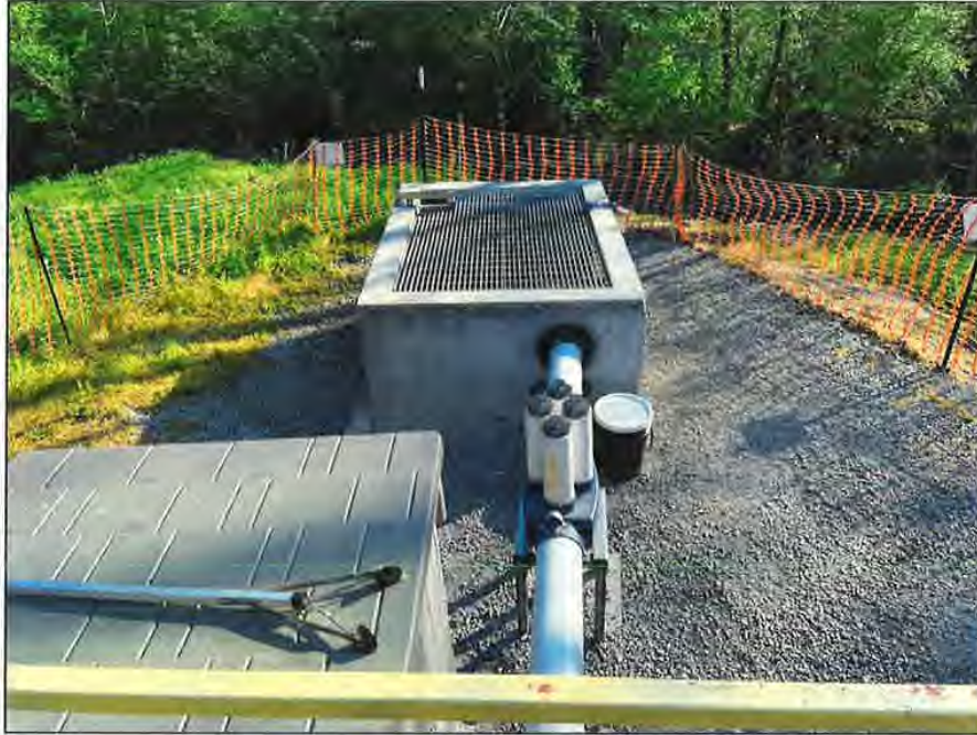
Chlorine Contact Basin
