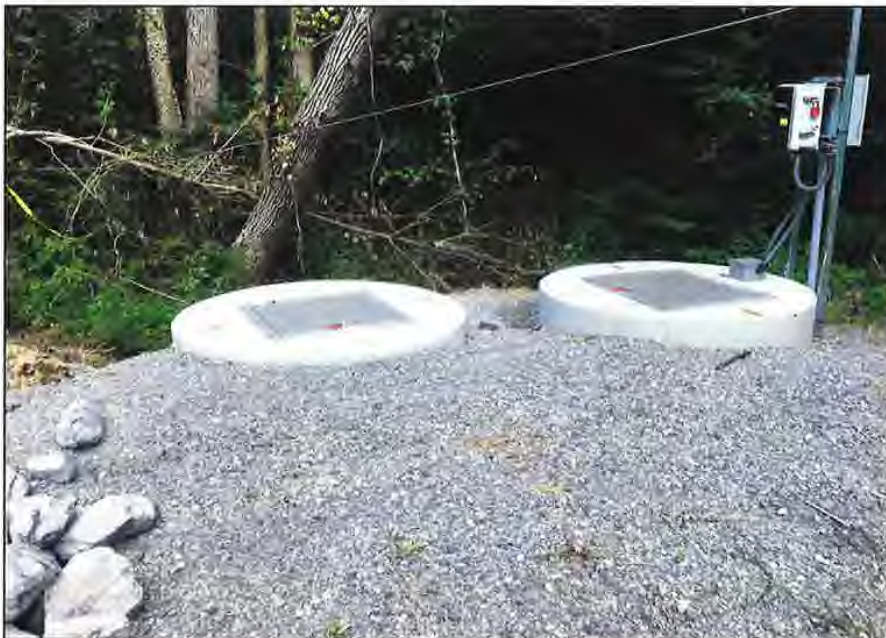
Mitchell Drive Lift Station – After Replacement
