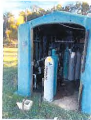
Gaseous Chlorine Storage
