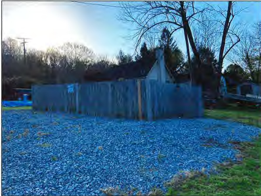
Herrington Haven WWTP
