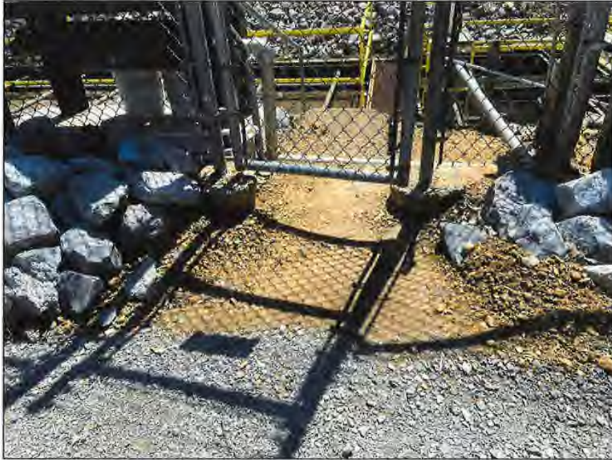
Gap under entrance gate
