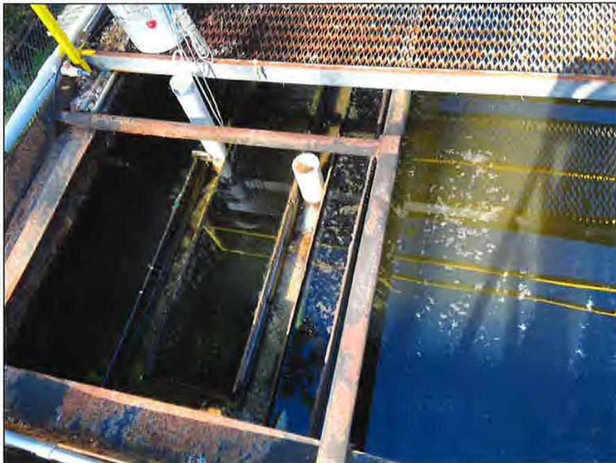
Clarifier and Weir Trough
