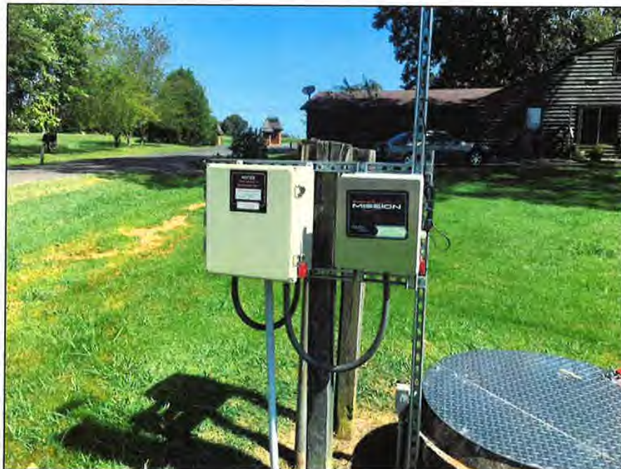
Remote Monitoring System
