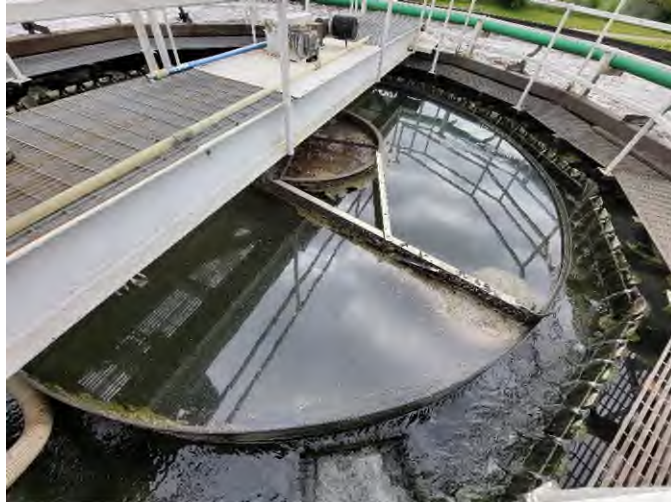
Notable solids passing through clarifier.
