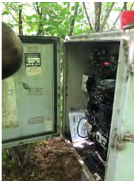
Unsafe wiring in the lift station control box.
