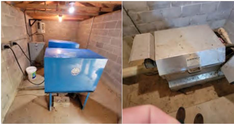
9 10 Blowers and tertiary filter in blower building.
