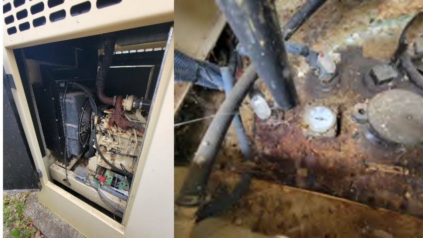
Rust and damage to the interior of the on-site generator.
