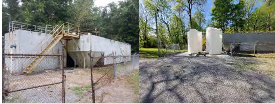
Tanks before and after repair and painting, new digester tanks on concrete pad.
