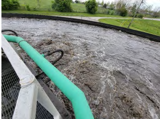
Coarse air diffusion pattern in aeration basins.
