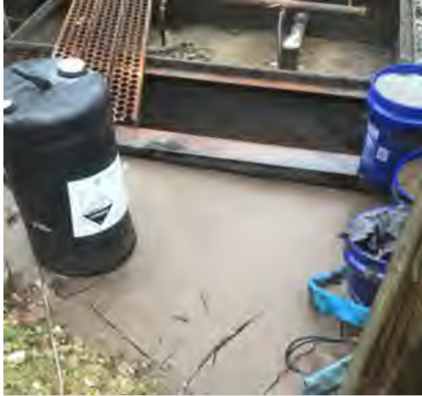
Sludge accumulation inside of fenced area around plant due to plant overflow.
