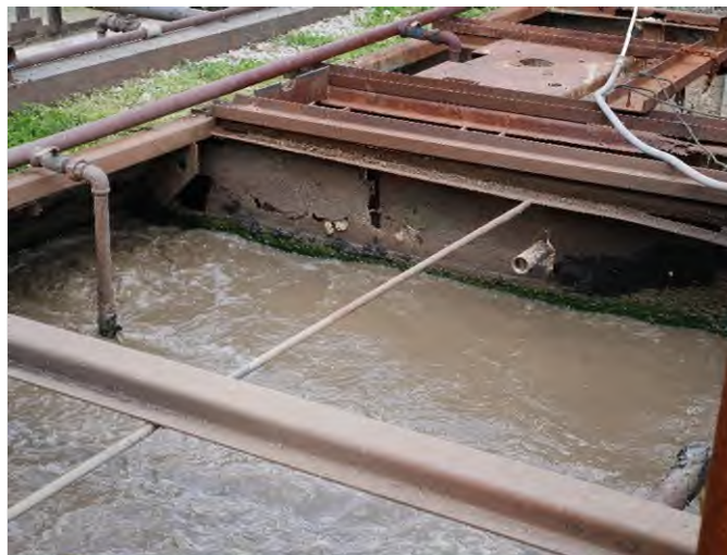
11 12 Coarse aeration pattern and severe rust in aeration basin.
