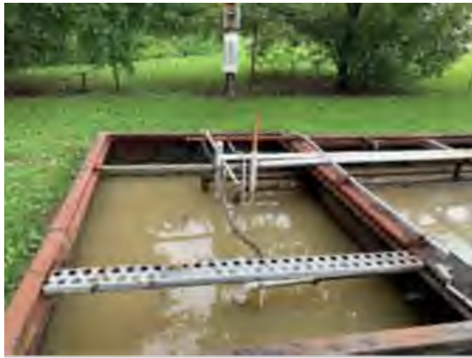
5 6 Woodland Acres treatment basin during a rainstorm. 7
