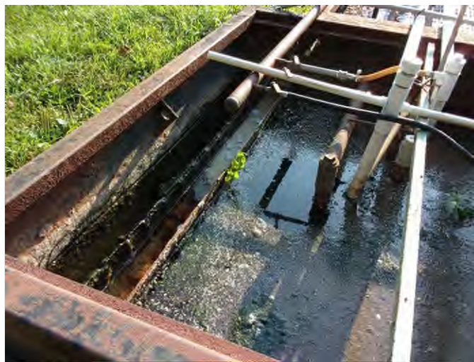
Woodland Acres clarifier.
