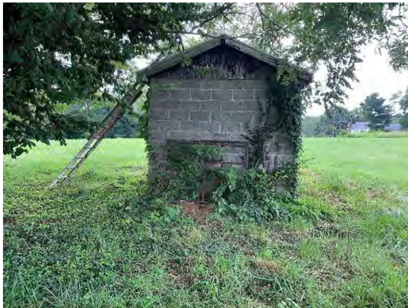
Overgrowth on control structure.
