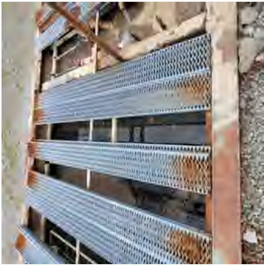
5 Rusted grating and tanks at time of acquisition.
