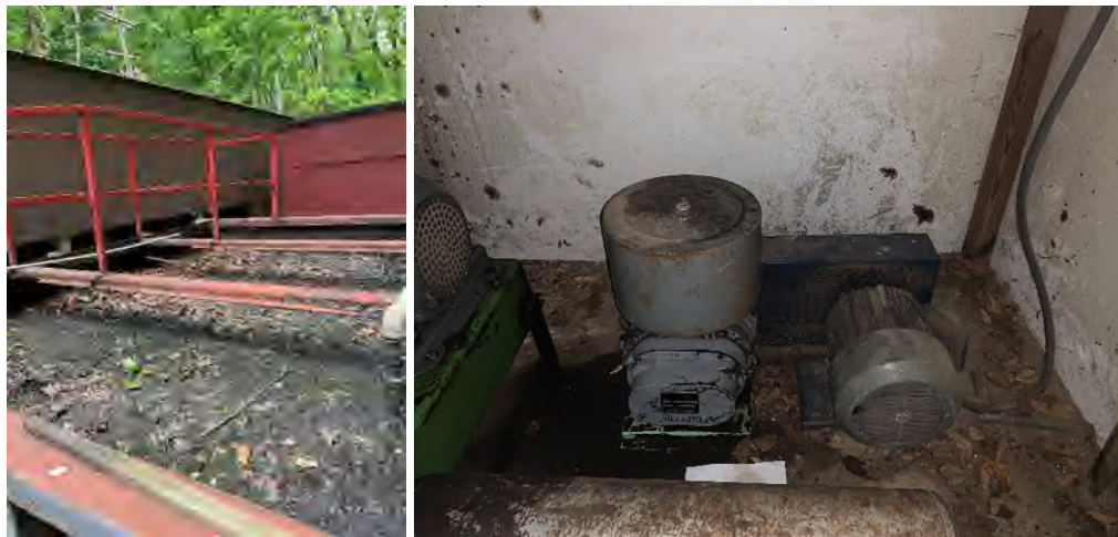
8 9 Sludge-holding tank full of impacted sludge and damaged blowers.
