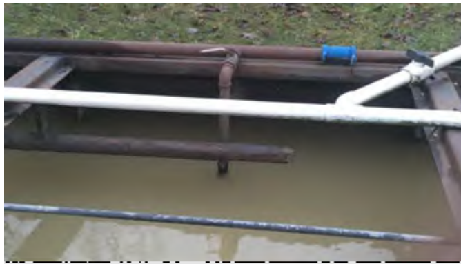
9 10 Broken sludge return pipe.
