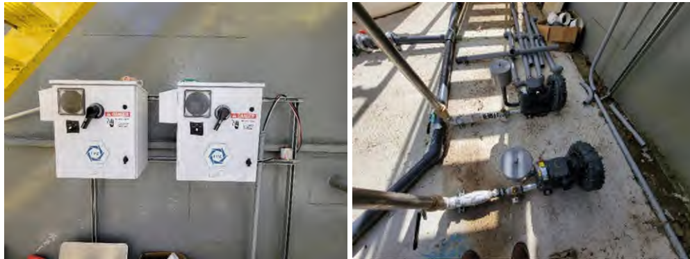
New blowers and controls for replacement digester system.
