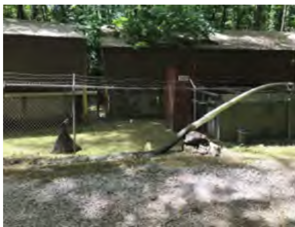
Improper influent line installation.
