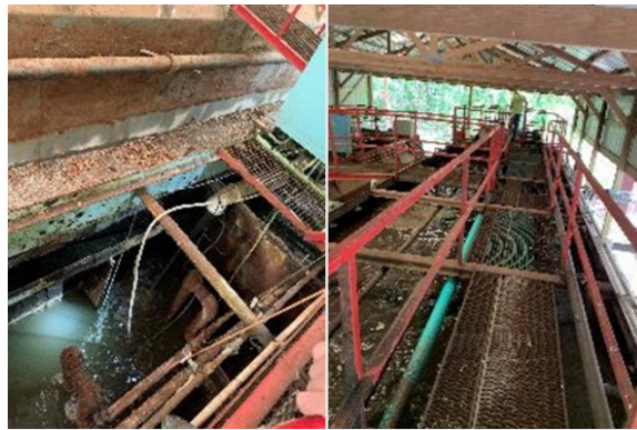
14 Severe corrosion and rust found throughout the River Bluffs facility. 15 16
