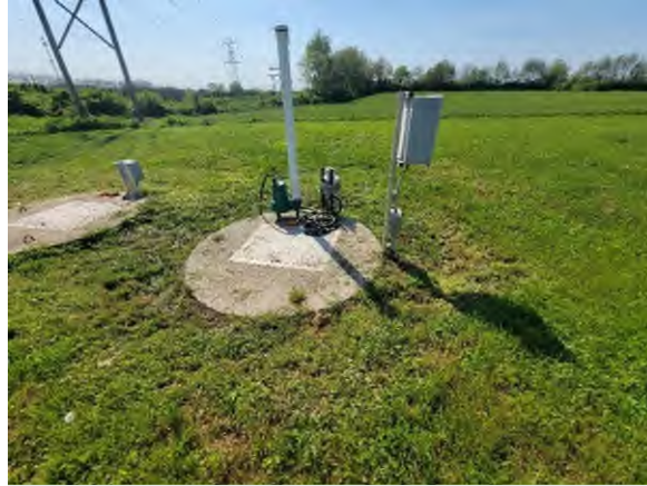
Small blower and control panel installed at wet well basins.
