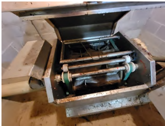
Damaged membrane on interior of tertiary filter.
