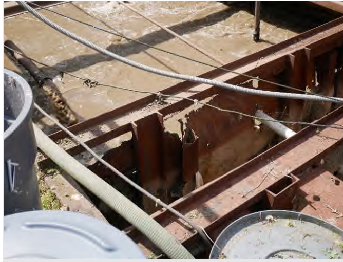
4 5 Woodland Acres steel tank deterioration. 6
