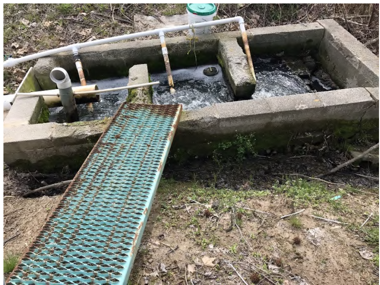
Chlorination Contact Chamber not up to code
