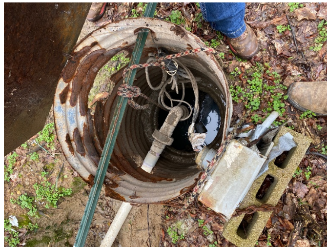
Non-standard/failing lift station 2
