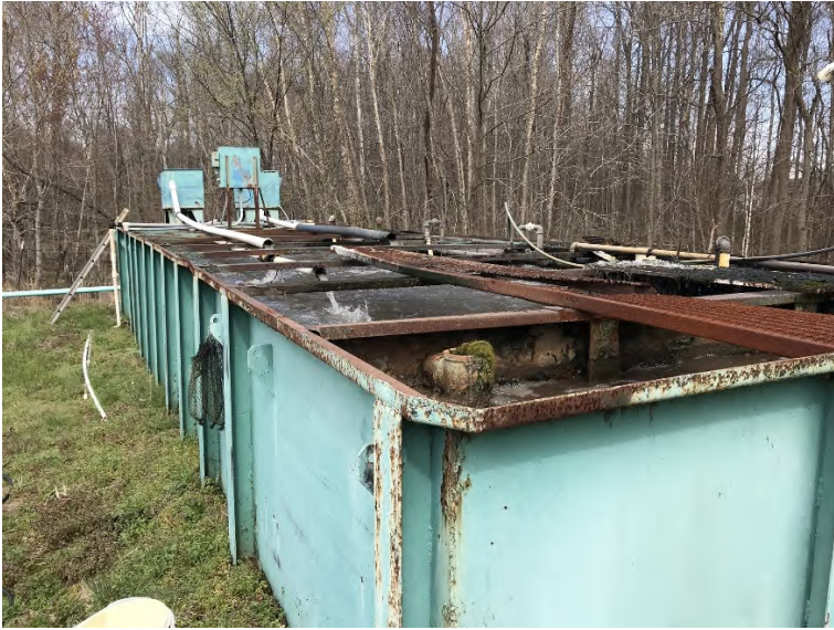
Activated Sludge – Extended Aeration tank beginning to rust/fail
