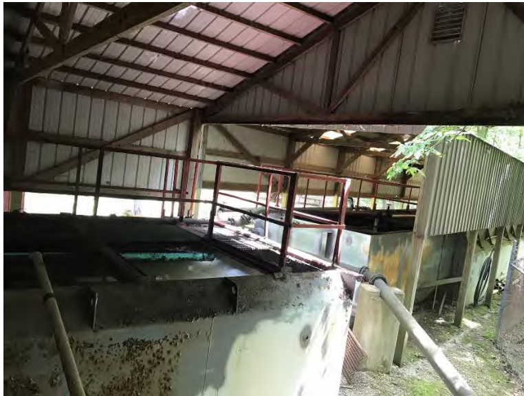
Treatment Tanks are rusting and have gone unmaintained
