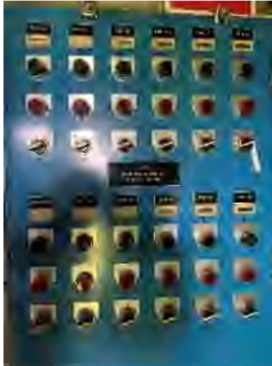
Irrigation Pump Stations Control Panel
