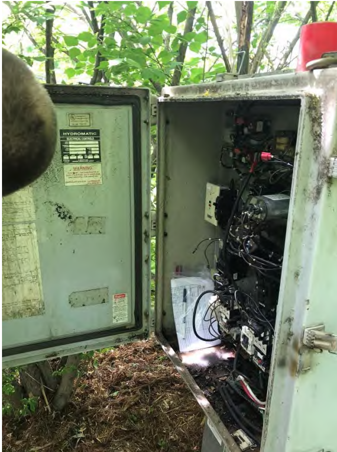
Lift station control panels appear to be poorly wired and are a safety concern.
