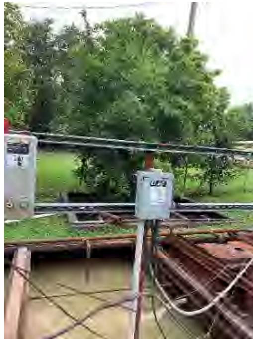
Electrical Boxes and Electrical Cabling
