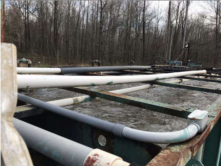
PVC lines need to be replaced
