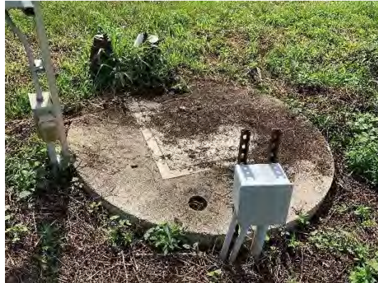
Triplex Irrigation Pump Station No. 1
