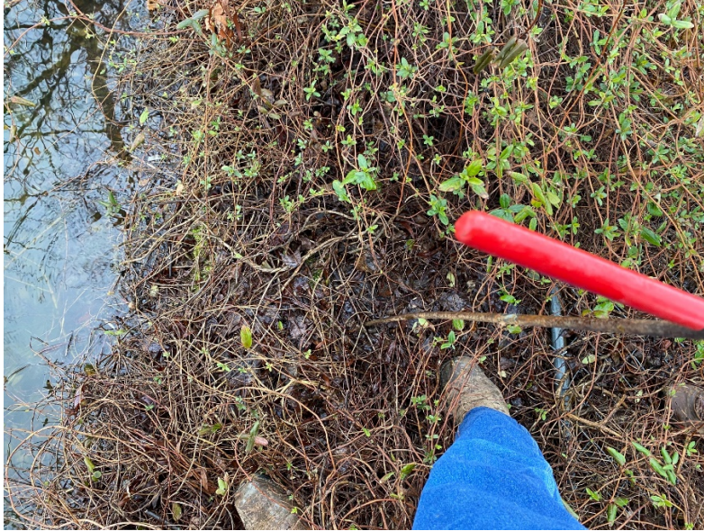
Lagoon Berm vegetation and sewage overflow
