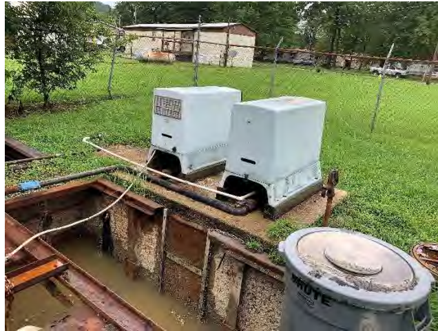
Blowers, EQ Basin, and Electrical Cables
