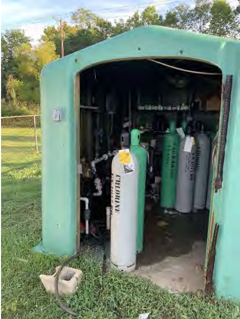
Gaseous Chlorine Storage
