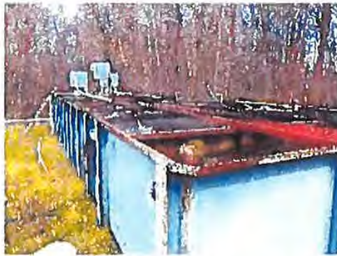
Activated Sludge - Extended Aeration tank beginning to rust/fail
