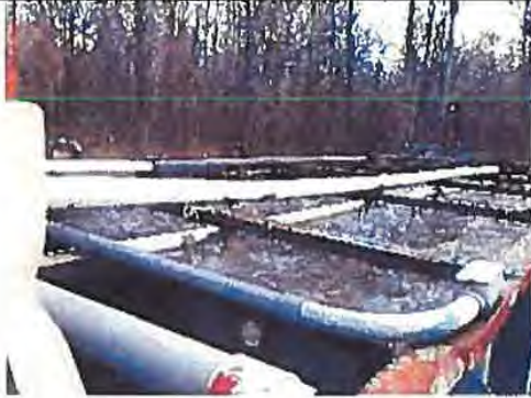
PVC lines need to be replaced
