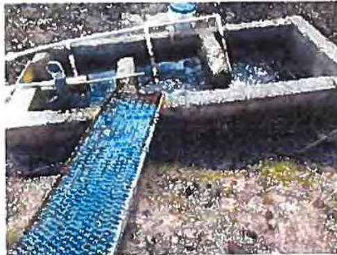
Chlorination Contact Chamber not up to code
