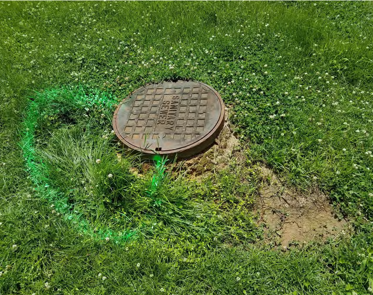
Sunken area around manhole. Corner of Golden Acres Loop and Kalee Dr.
