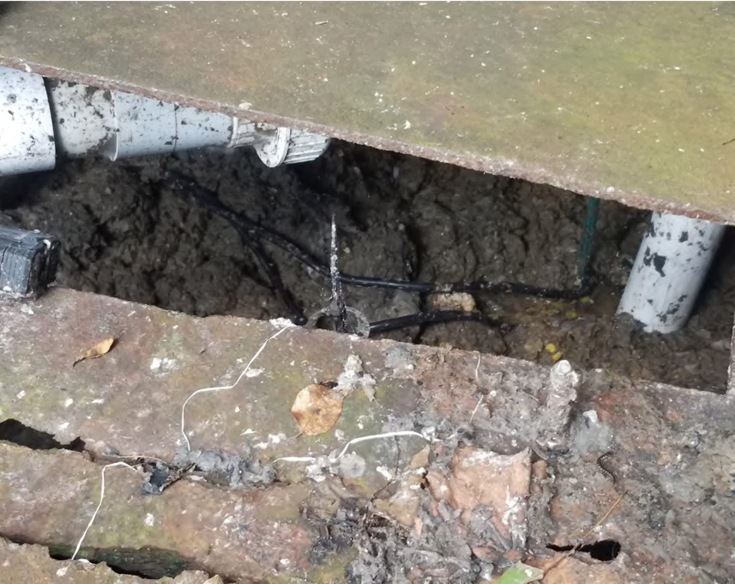
Lift station full of solids
