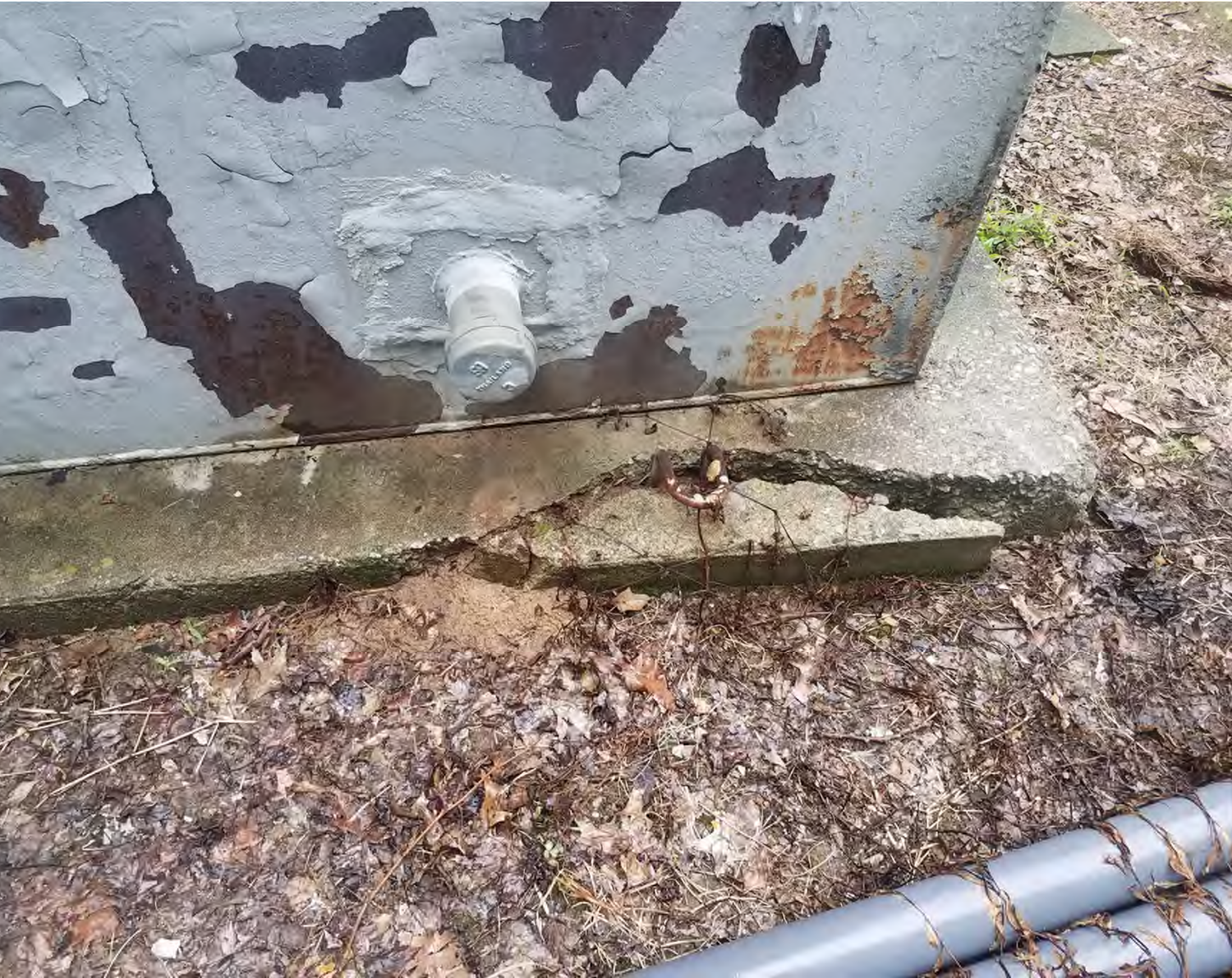
Crack in the foundation of the treatment plant
