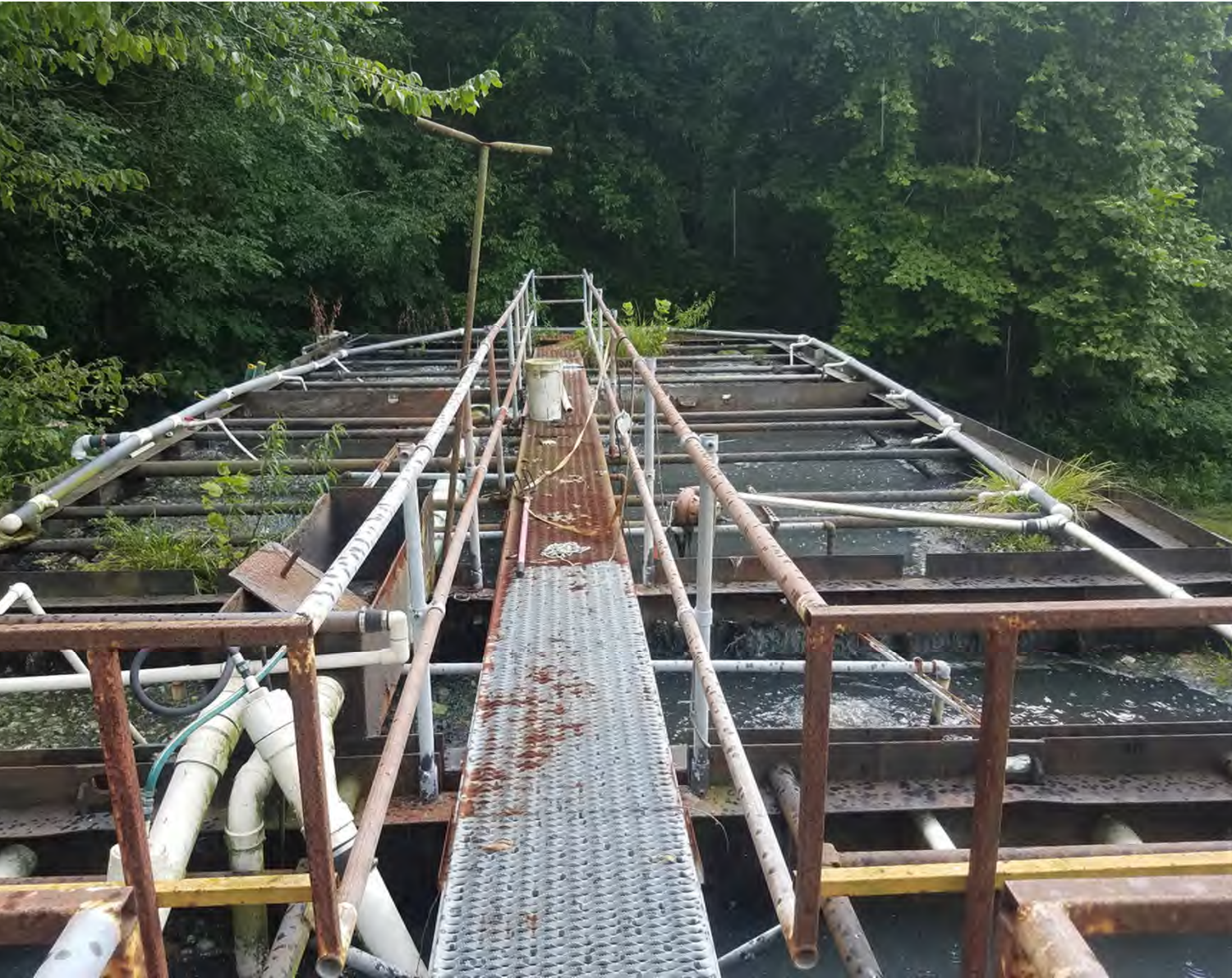
WW treatment plant
