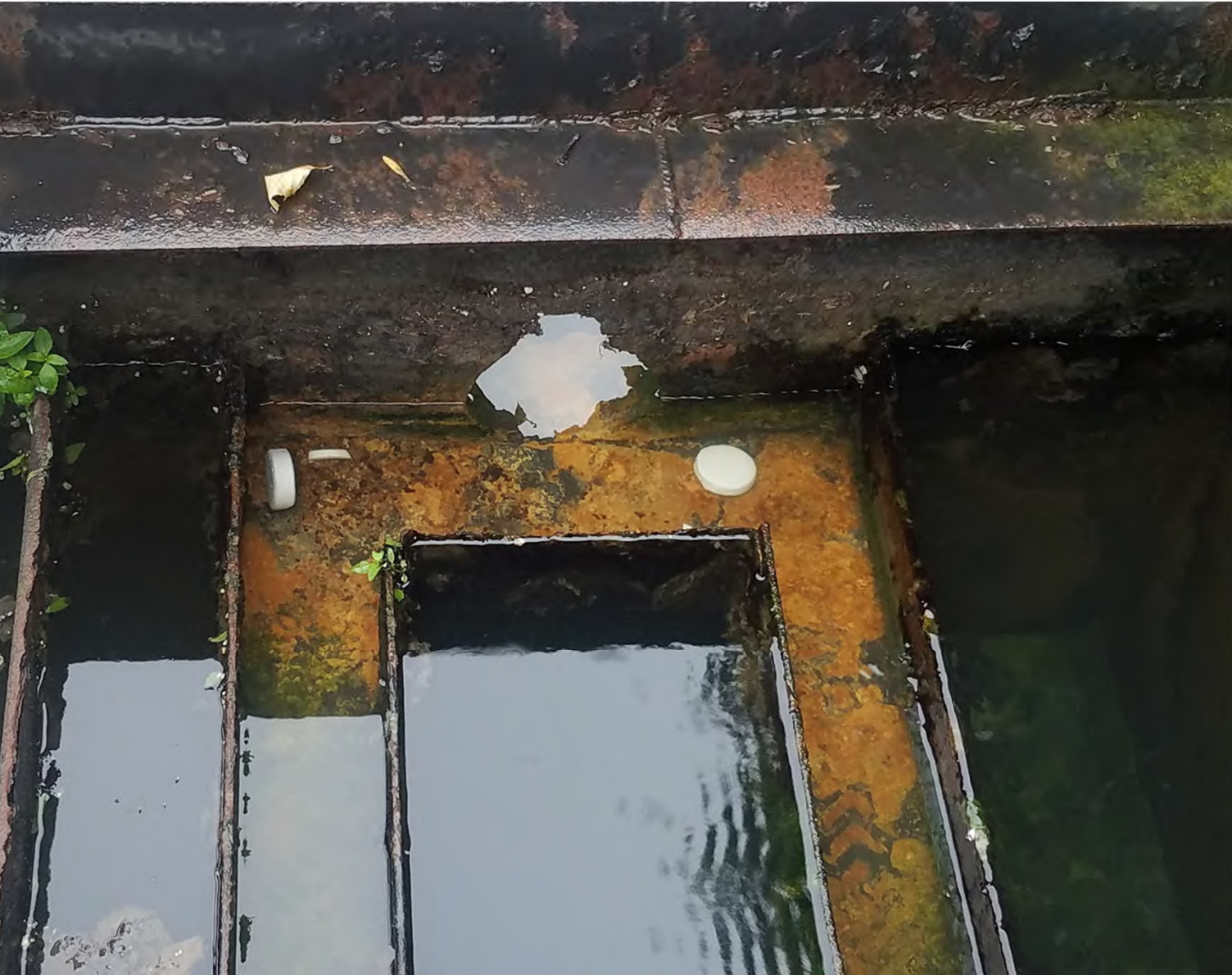
Cl2 tablets in place
