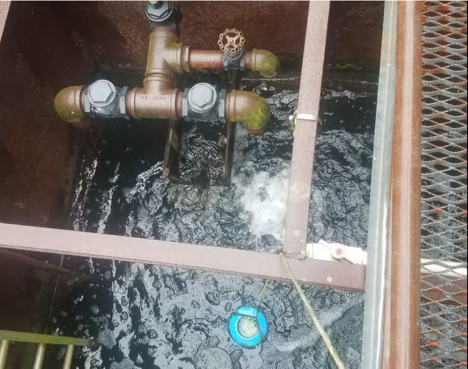
Contact chamber discharge
