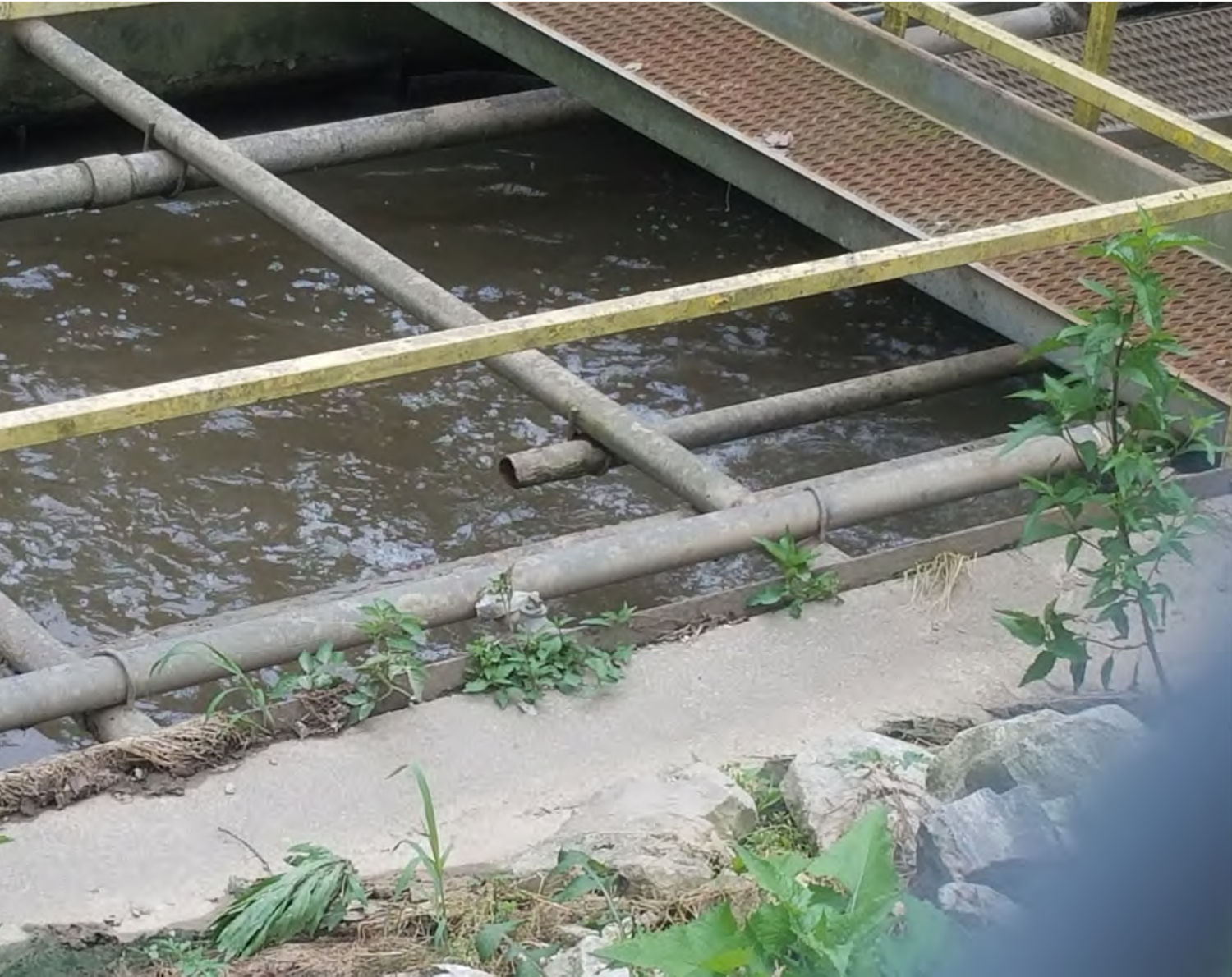
Sludge return discharge
