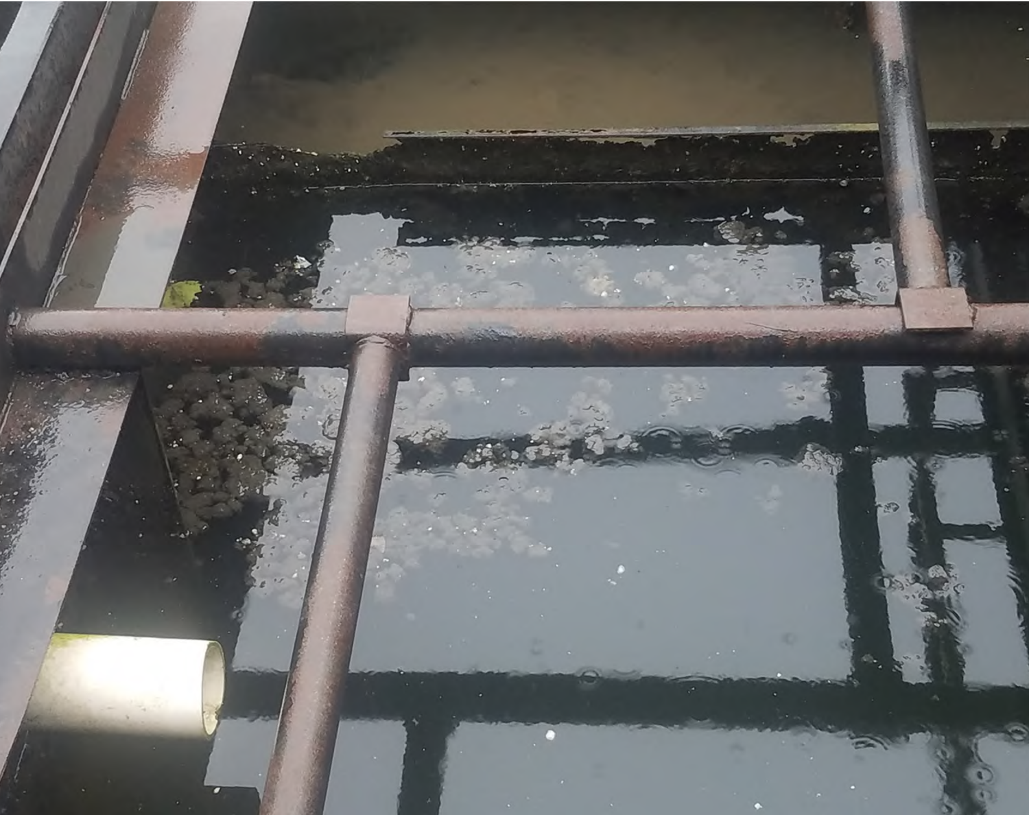
Solids floating in the clarifier
