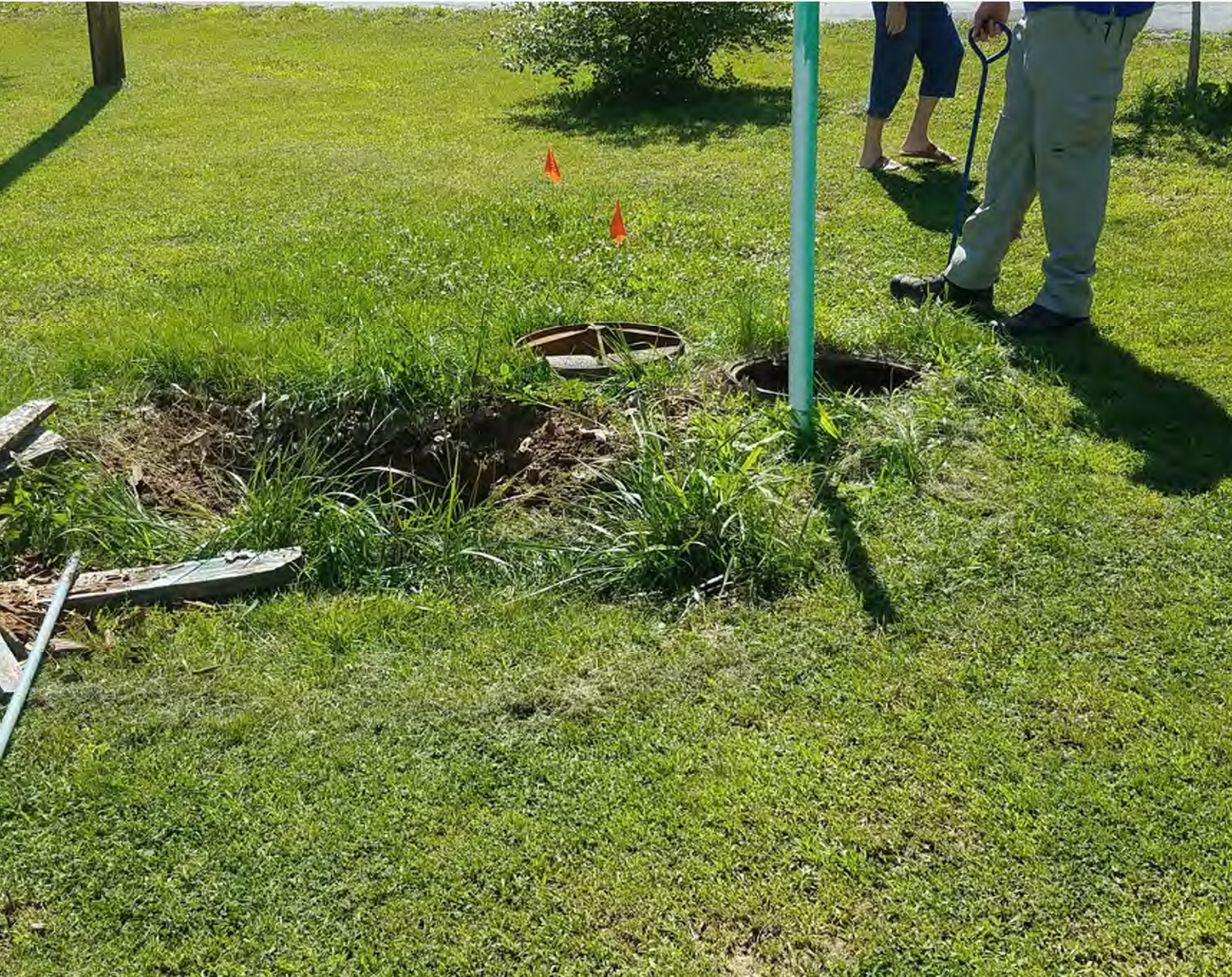
Sunken area near manhole. 8957 US HWY 68.
