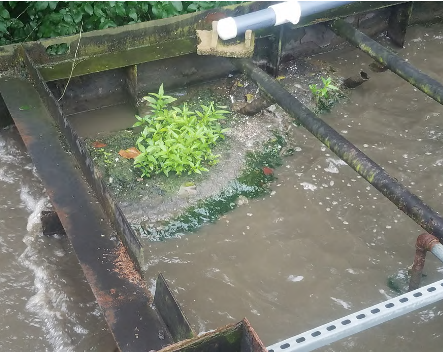
Solid mass in aeration chamber
