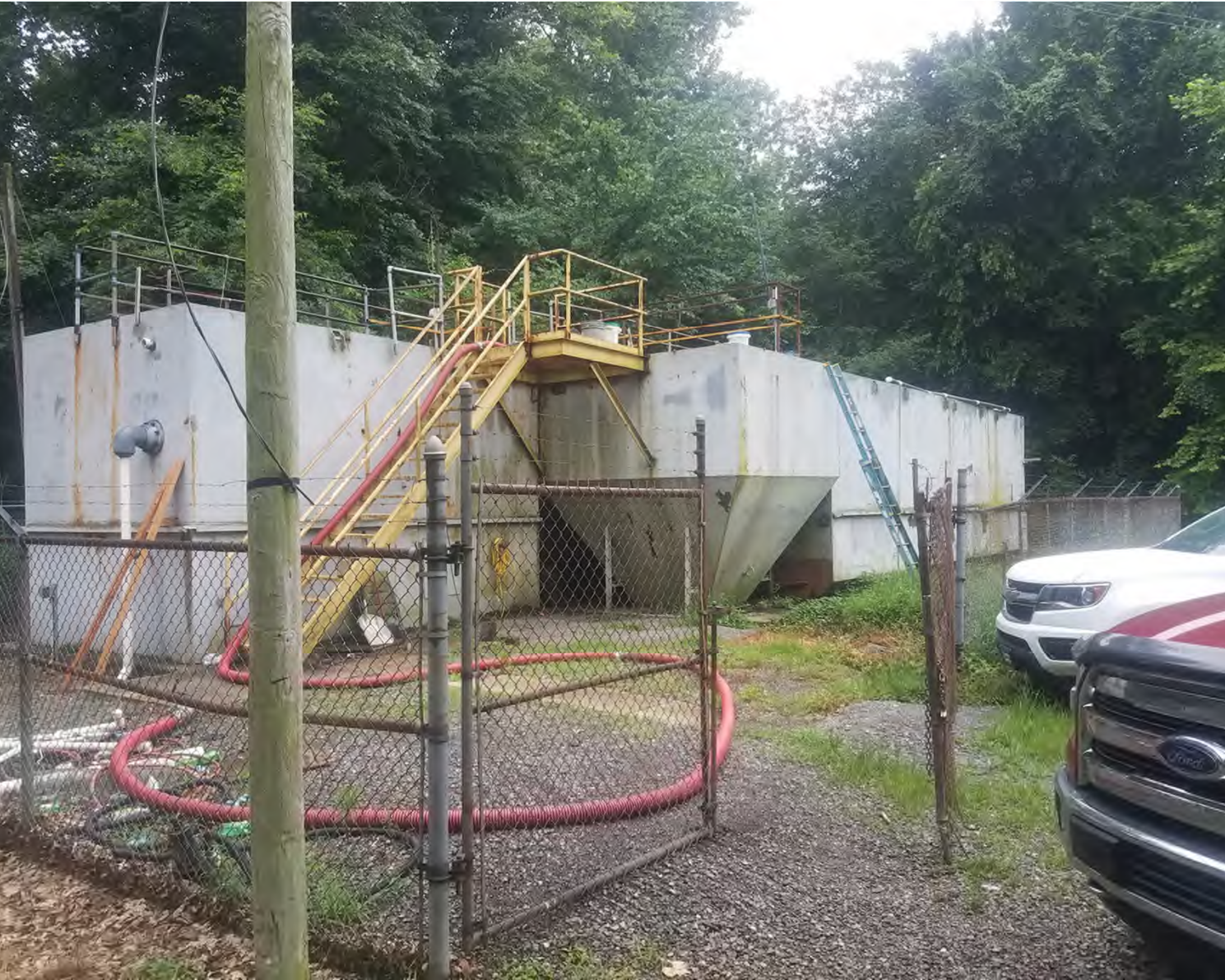
WW treatment plant
