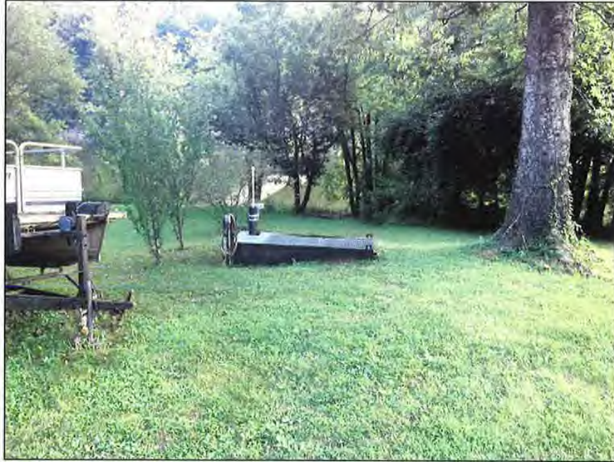
Chlorine Contact Tank
