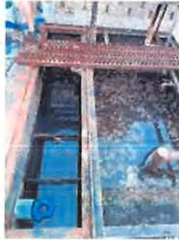
Clarifier and Contact Tank
