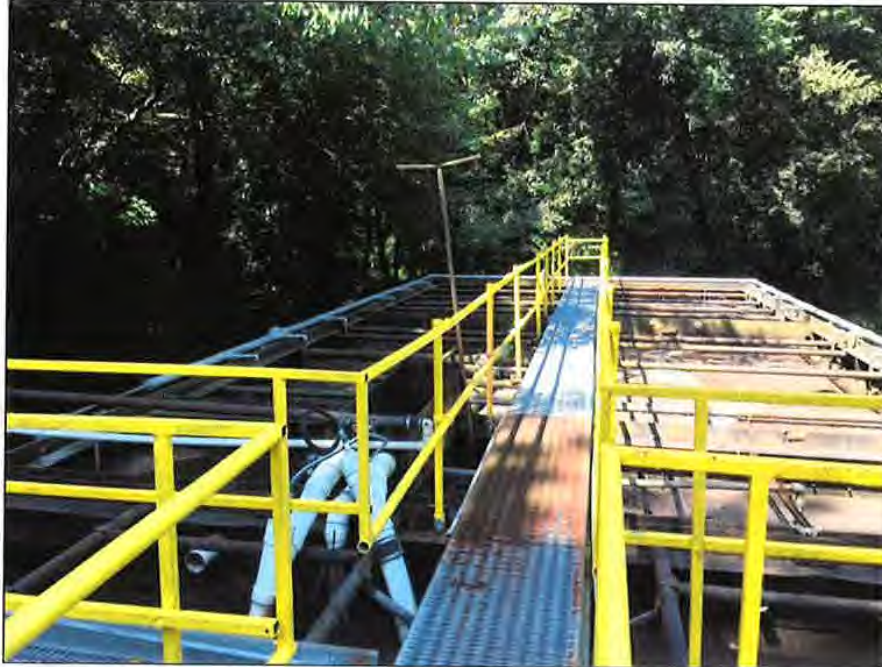
Top View of the Plant
