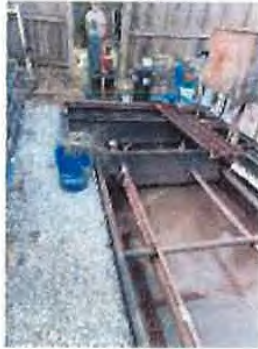
Aeration Tank, Clarifier, Contact Tank
