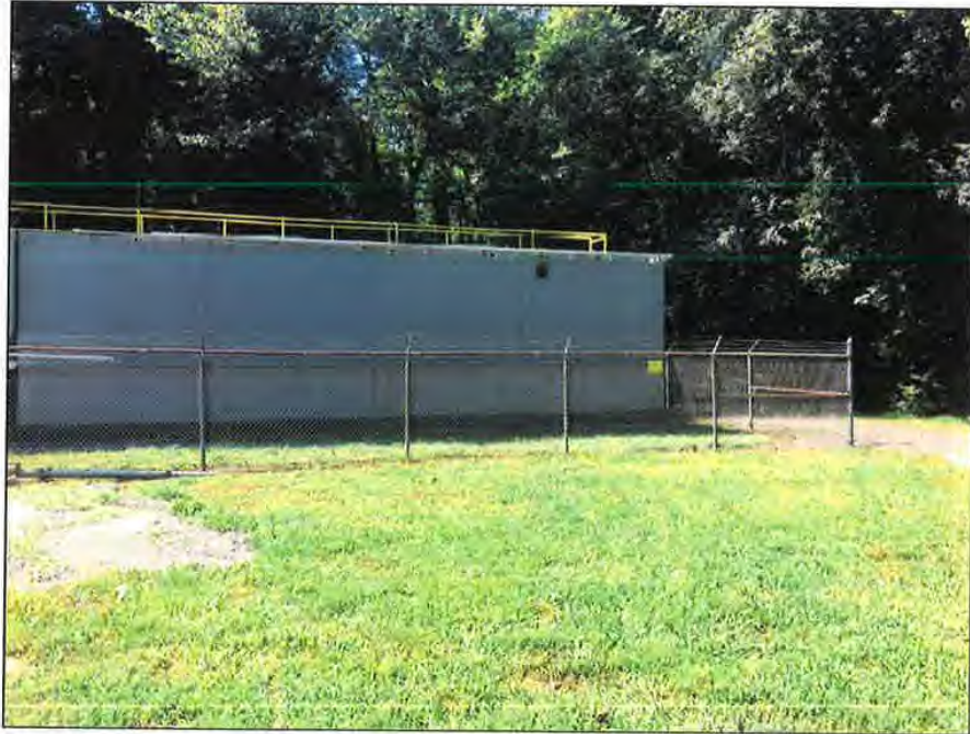
Great Oaks WWTF
