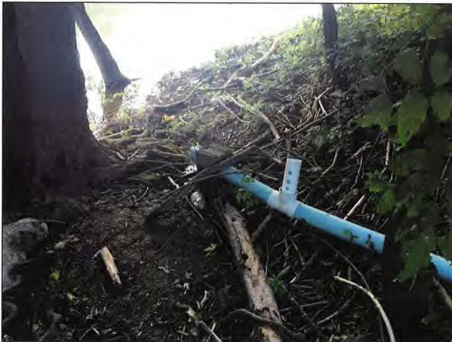
De-chlorination Dispenser and the Effluent Outfall
