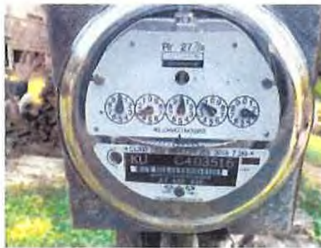
WWTP Electrical Meter
