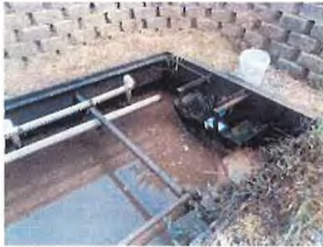
Manually Cleaned Bar Screen
