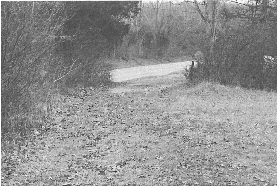
Photo shows the condition of access road. The access road was found to be in good condition at the time of inspection.
