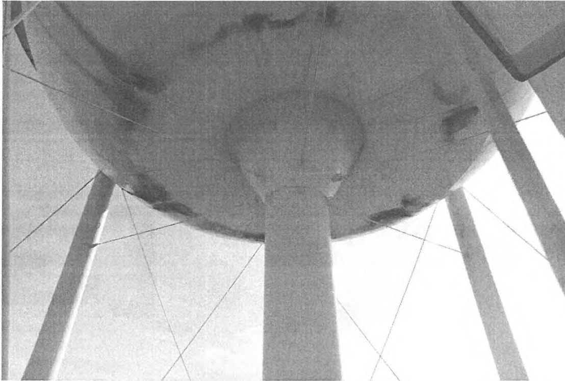
Photo shows the condition of the riser pipe and bowl. The connection appears to be in good condition.
