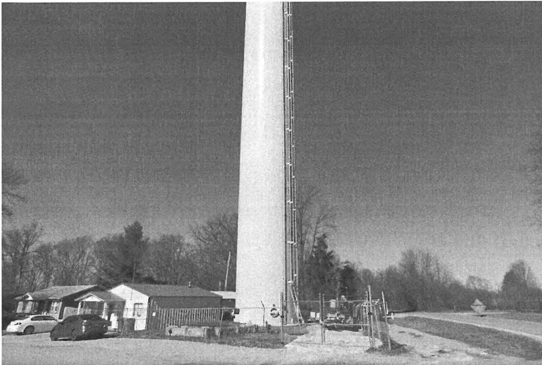
Photo shows the condition of access road. The access road was found to be in good condition at the time of inspection.
