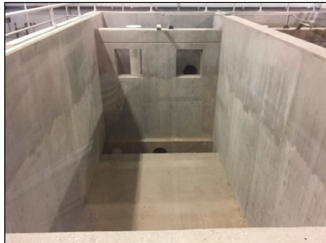
Figure #5– Filter No. 4 (Out-of-Service)
