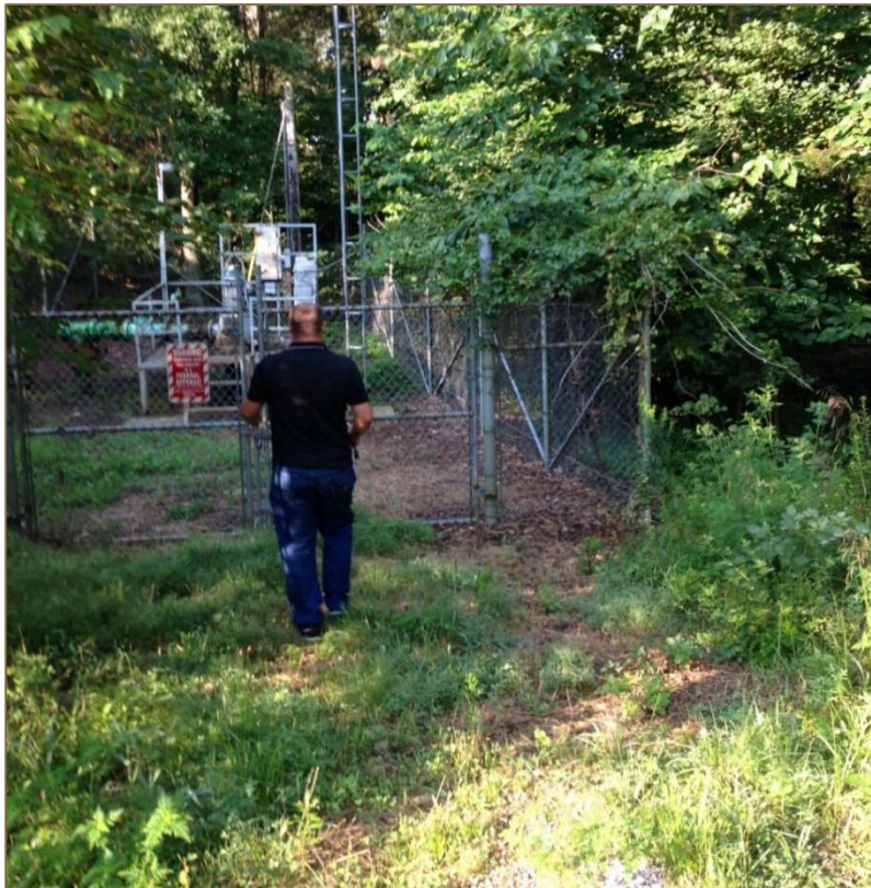
Figure #1 – Existing Gray Lane Raw Water Pump Station
