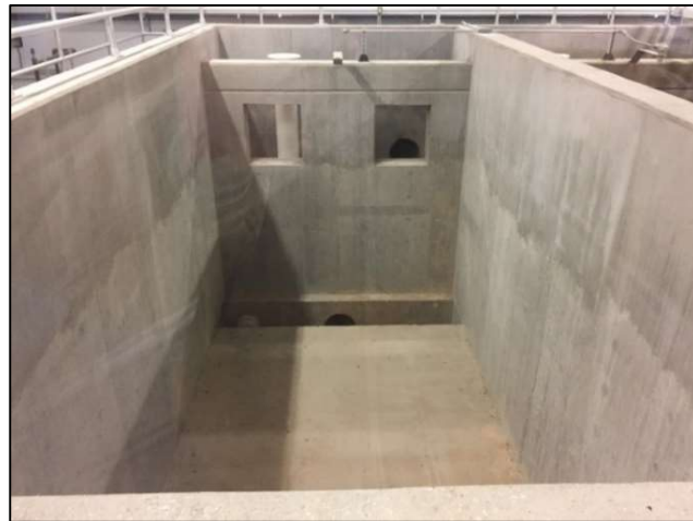
Figure #5 – Filter No. 4 (Out-of-Service)
