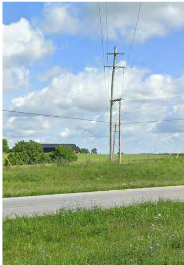
Figure 8: Looking south from Duncannon Lane at the existing 69kv EKPC Circuit (Google Street View Image)
