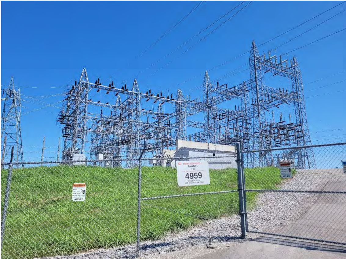
Figure 7: Fawkes Substation Starting Location (NV5 Field Photo)
