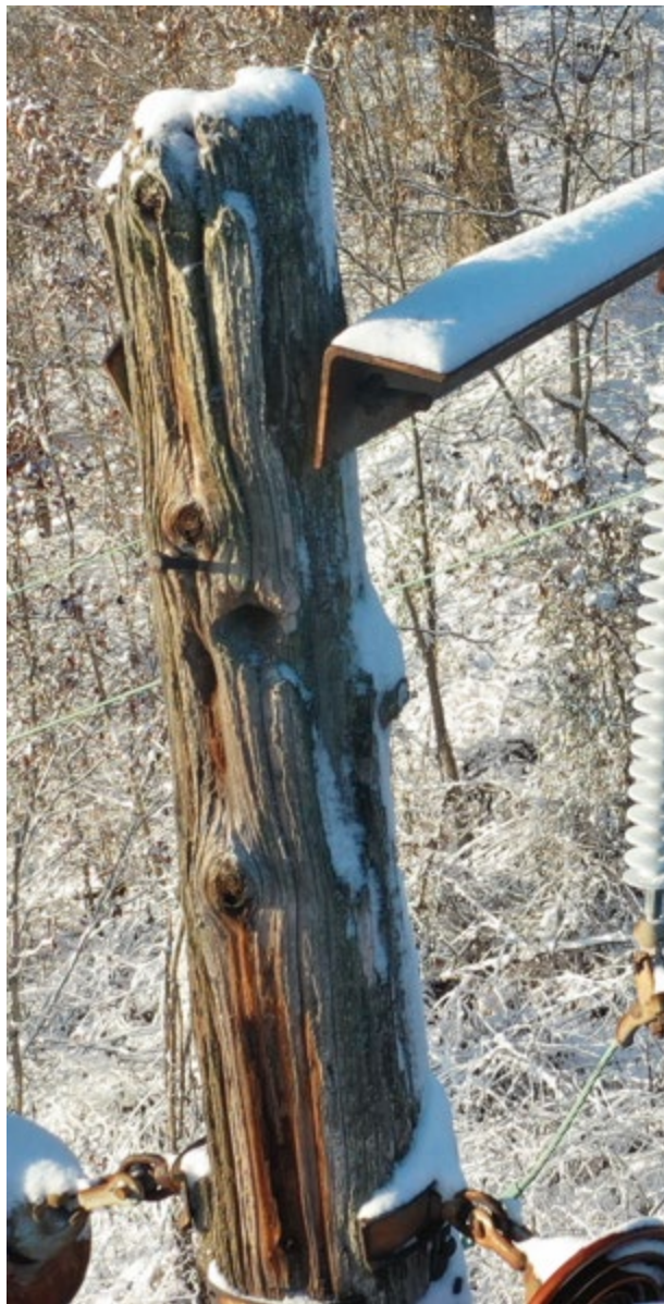
Structure K426-12: - Upper Pole Decay - Pole Cavities
