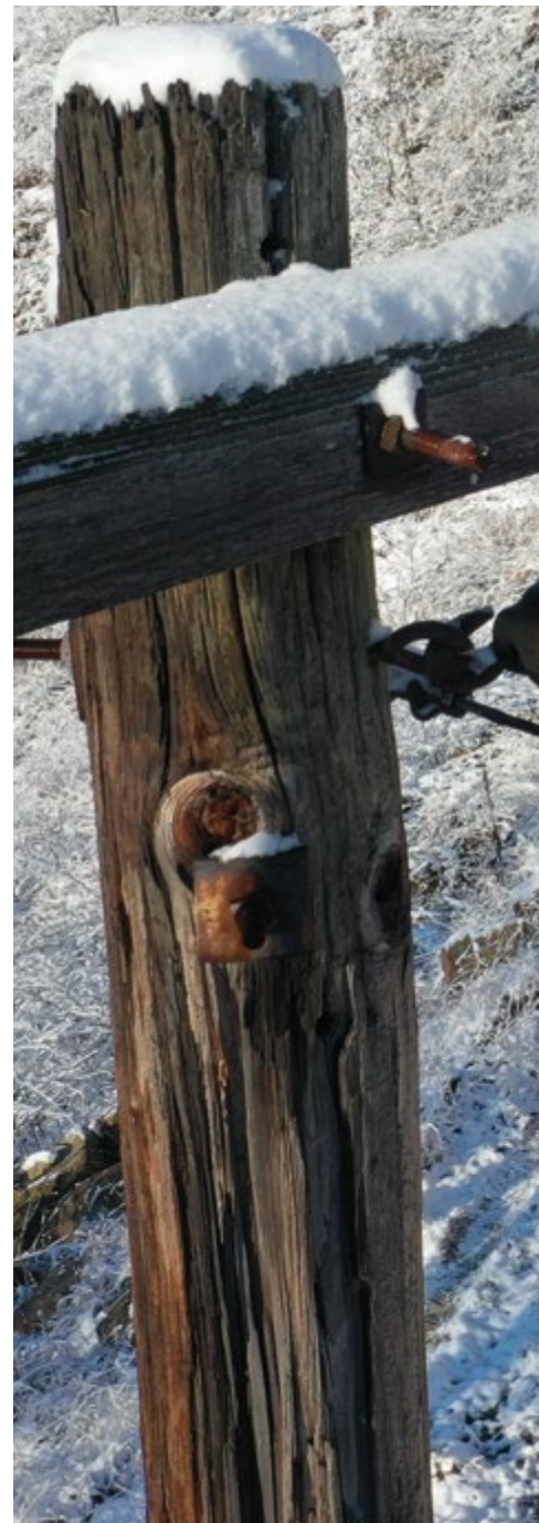
Structure K426-37: - Upper Pole Splitting
