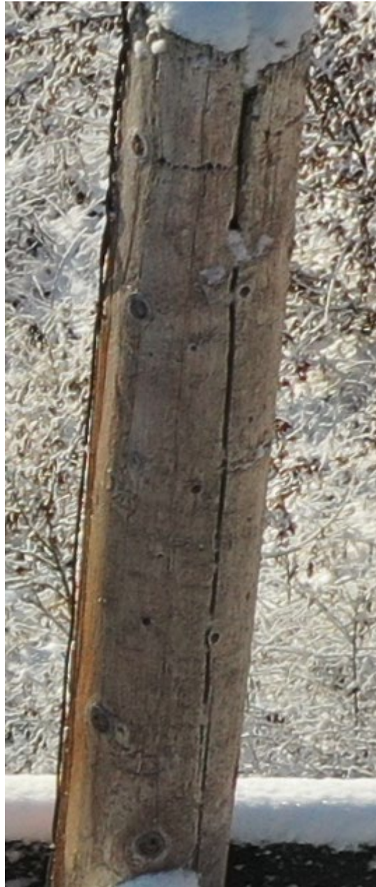
Structure K426-11: - Upper Pole Splitting
