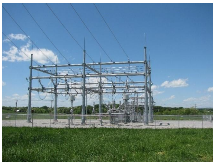
Figure 1: Comparable Proposed Substation
