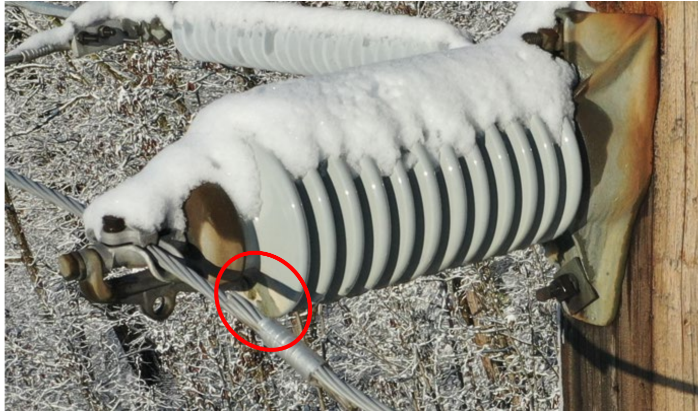
Structure K426-36: - Minor Insulator Flashover Evidence
