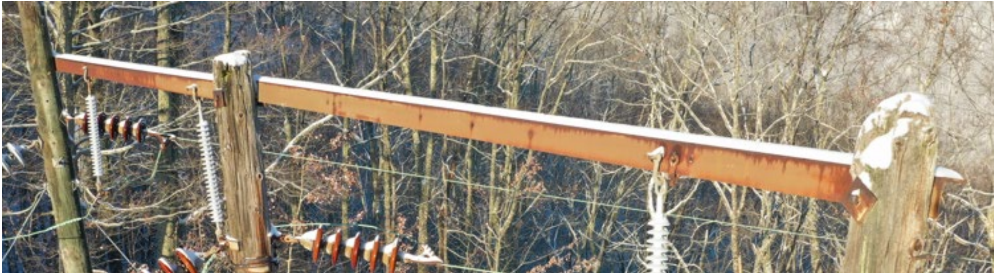
Structure K426-12: - Crossarm and Hardware Rusting
