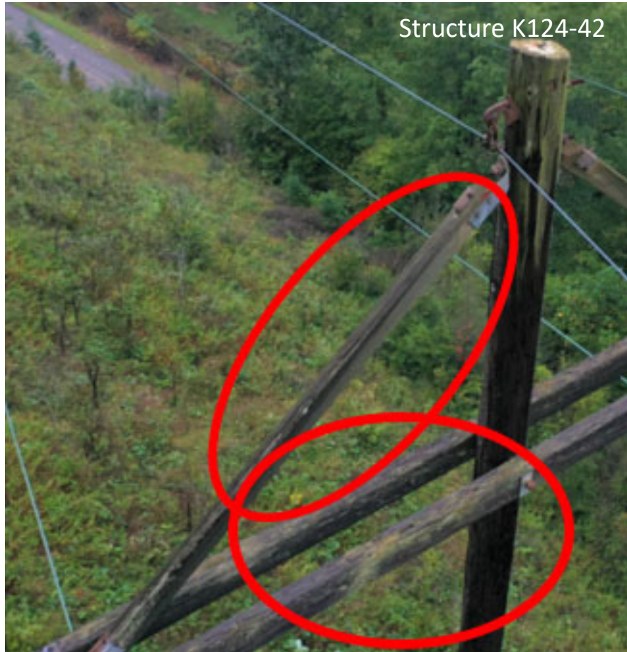
Structure K124-42: - Crossarm & Knee Brace Weathering
