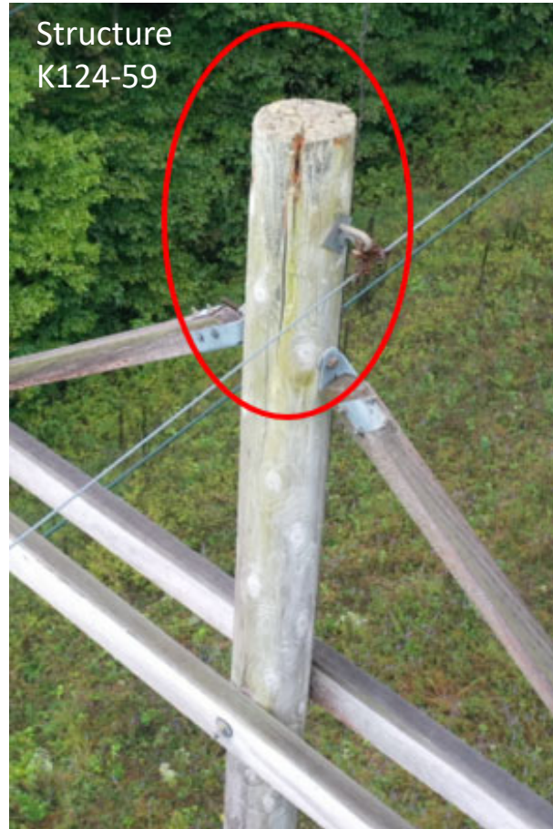
Structure K124-59: - Upper Pole Splitting
