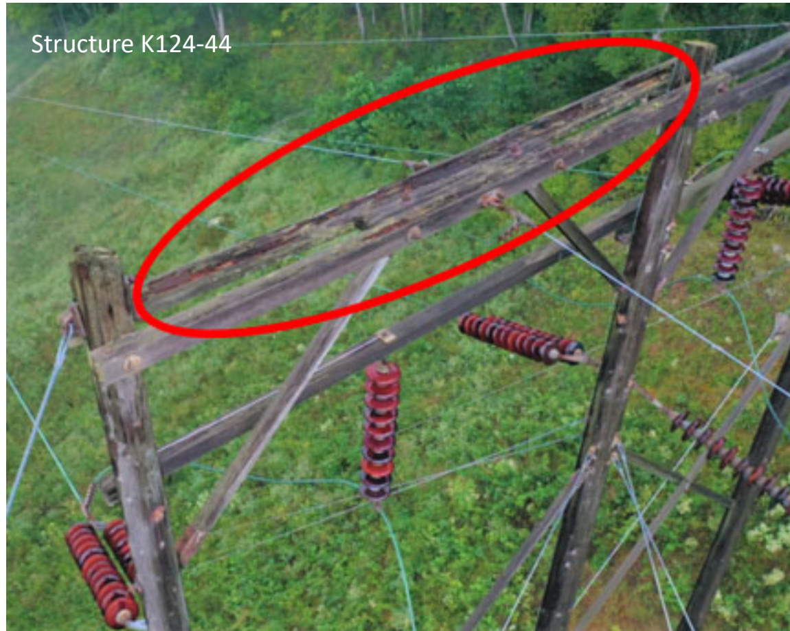
Structure K124-44: - Crossarm & Crossarm Block Splitting - Upper Pole Splitting
