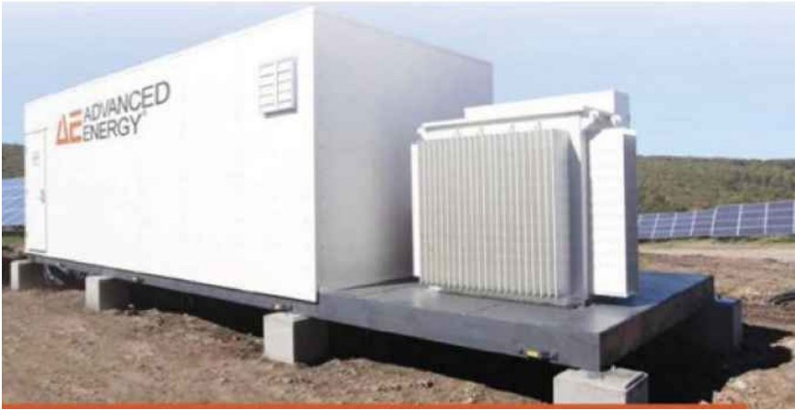
Inverter enclosure & medium voltage transformer
