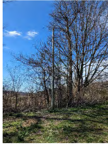
Photo 2: Typical transmission line pole located within the subject property
