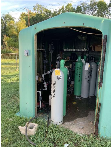
Gaseous Chlorine Storage
