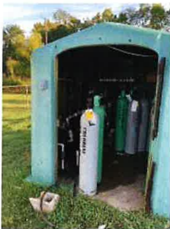
Gaseous Chlorine Storage
