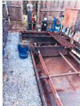
Aeration Tank, Clarifier, Contact Tank
