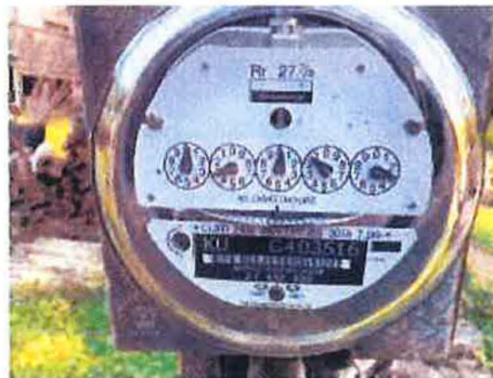
WWTP Electrical Meter
