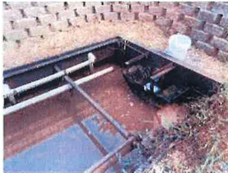
Manually Cleaned Bar Screen
