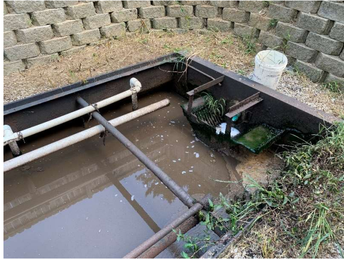
Manually Cleaned Bar Screen
