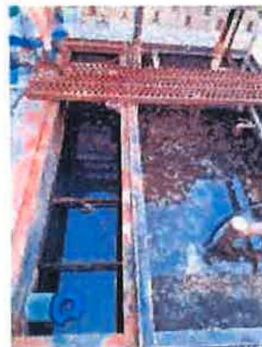
Clarifier and Contact Tank
