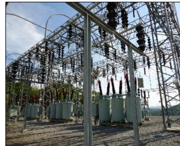
Cordell Hull Switchyard
