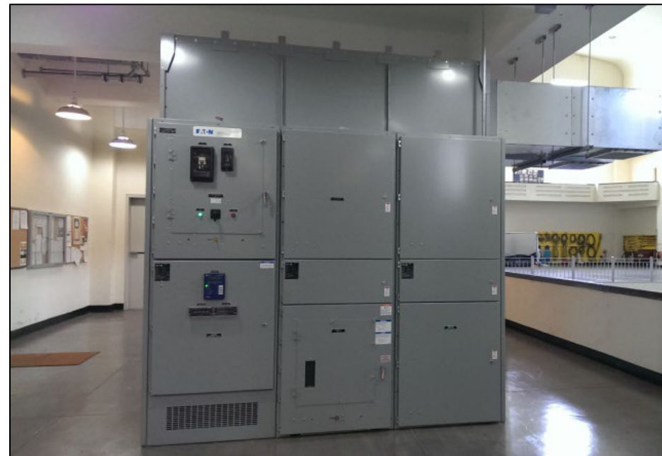
Generator Circuit Breaker at Center Hill
