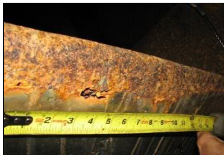
Cheatham Turbine Runner Cavitation Damage
