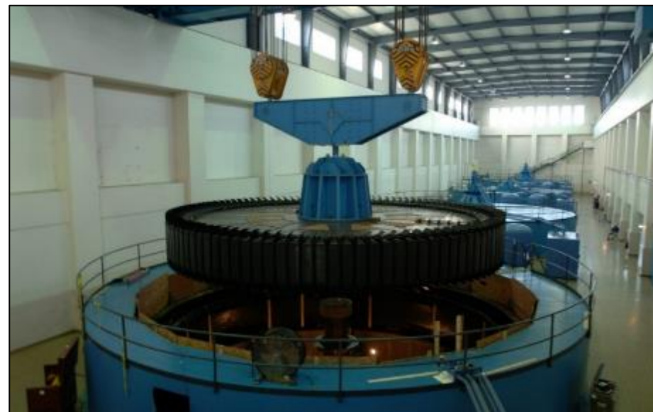
Barkley Unit #1 Rotor Removed for Refurbishment
