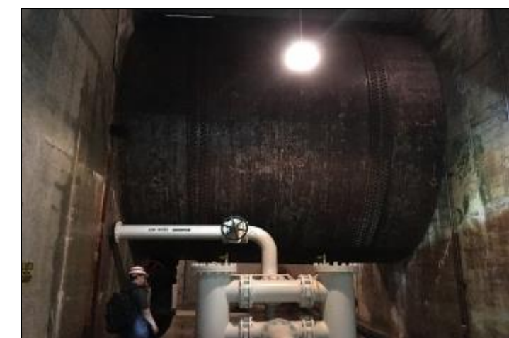
Center Hill Penstock
