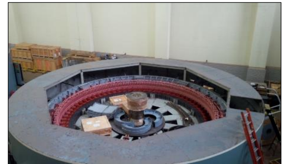
Refurbished Center Hill Unit #1 Generator
