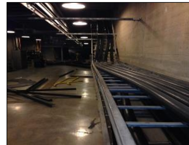
Barkley Medium Voltage Cables
