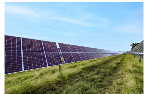
Solar panels are mounted on posts, enabling growth of vegetation underneath that allows for natural drainage and the interception of storm water
