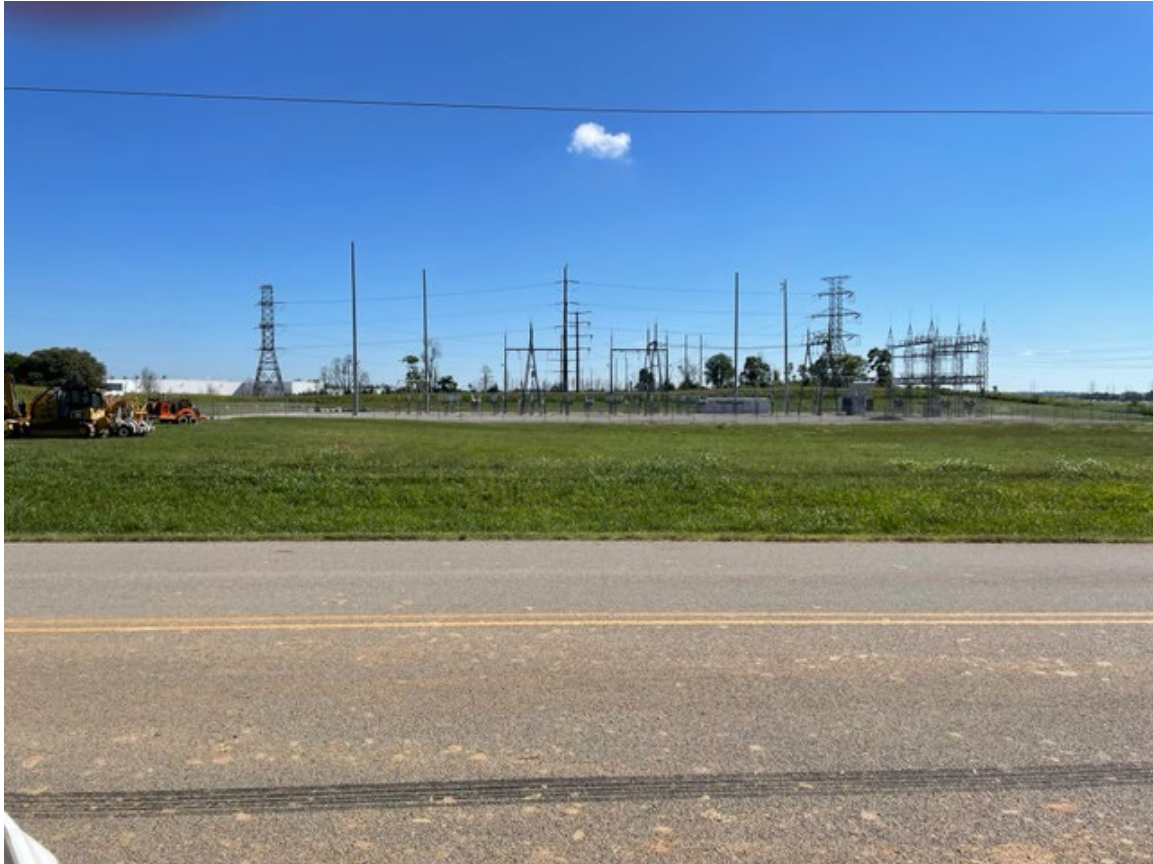
Figure C-15. EKPC substation across Hayden School Road from project substation
