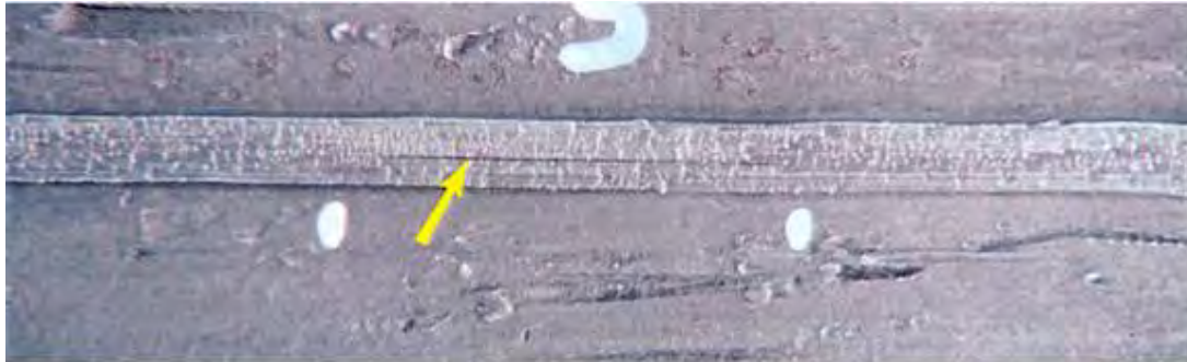
Photograph of Weld Seam ID Surface.
