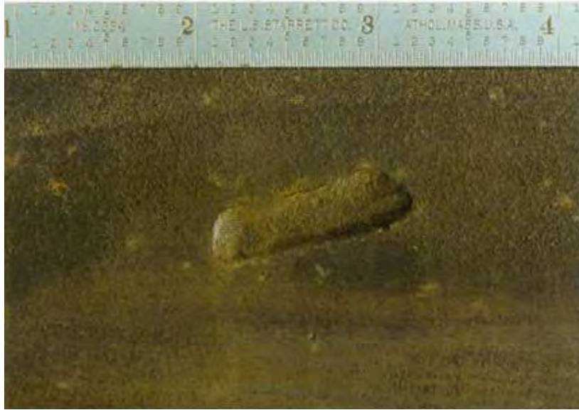
Photograph of ID Pipe Surface Near Seam Weld.
