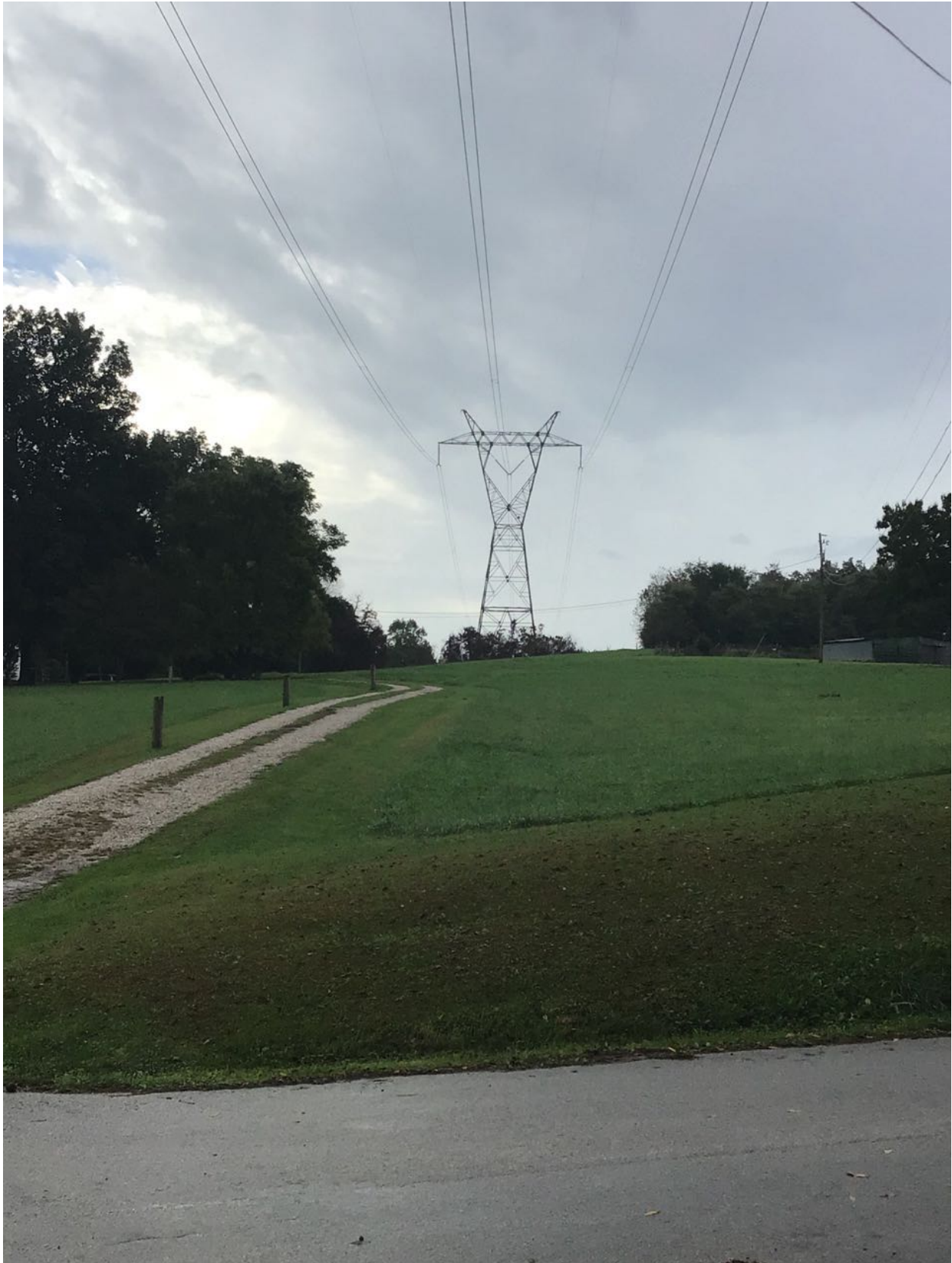
Figure 68 Existing 345 kV Brown North to Hardin County Transmission Line off W Rhudes Creek Road
