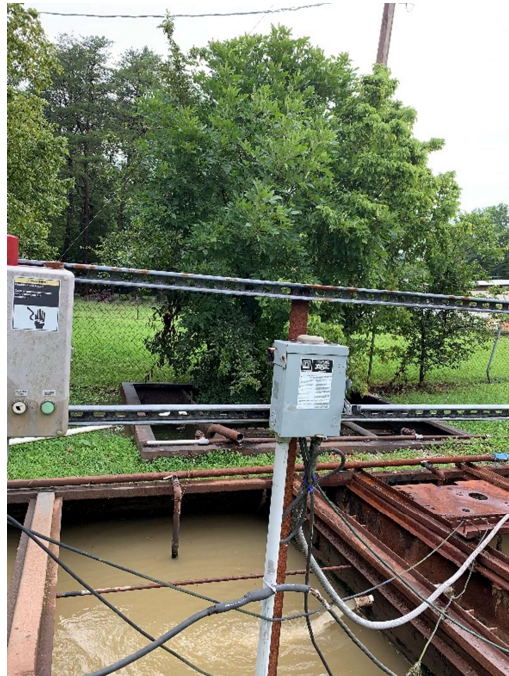
Electrical Boxes and Electrical Cabling
