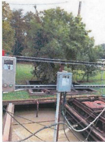
Electrical Boxes and Electrical Cabling
