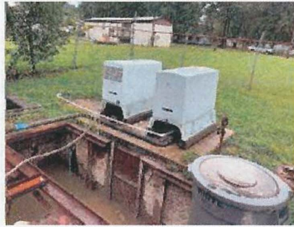
Blowers, EQ Basin, and Electrical Cables
