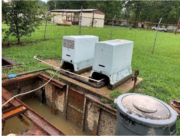
Blowers, EQ Basin, and Electrical Cables
