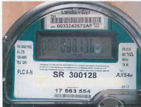
WWTP Electrical Meter
