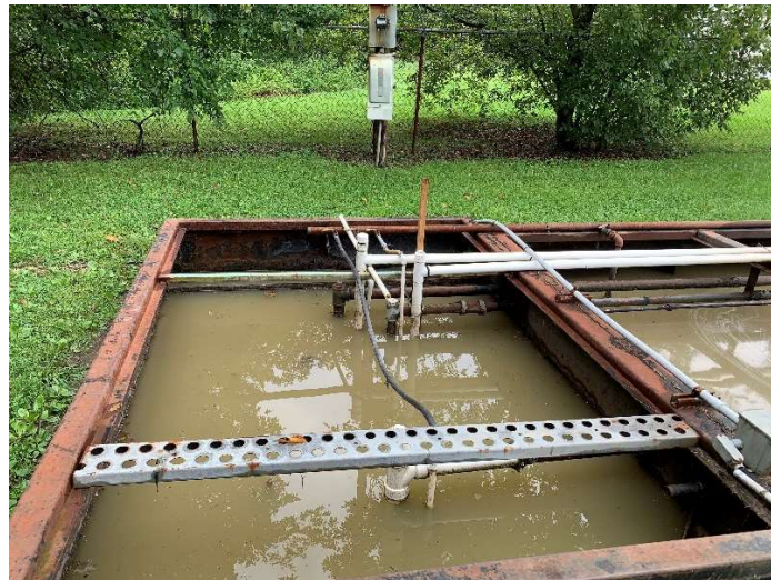
Clarifier Performance During Wet Weather (and No Aeration in Aeration Tank)
