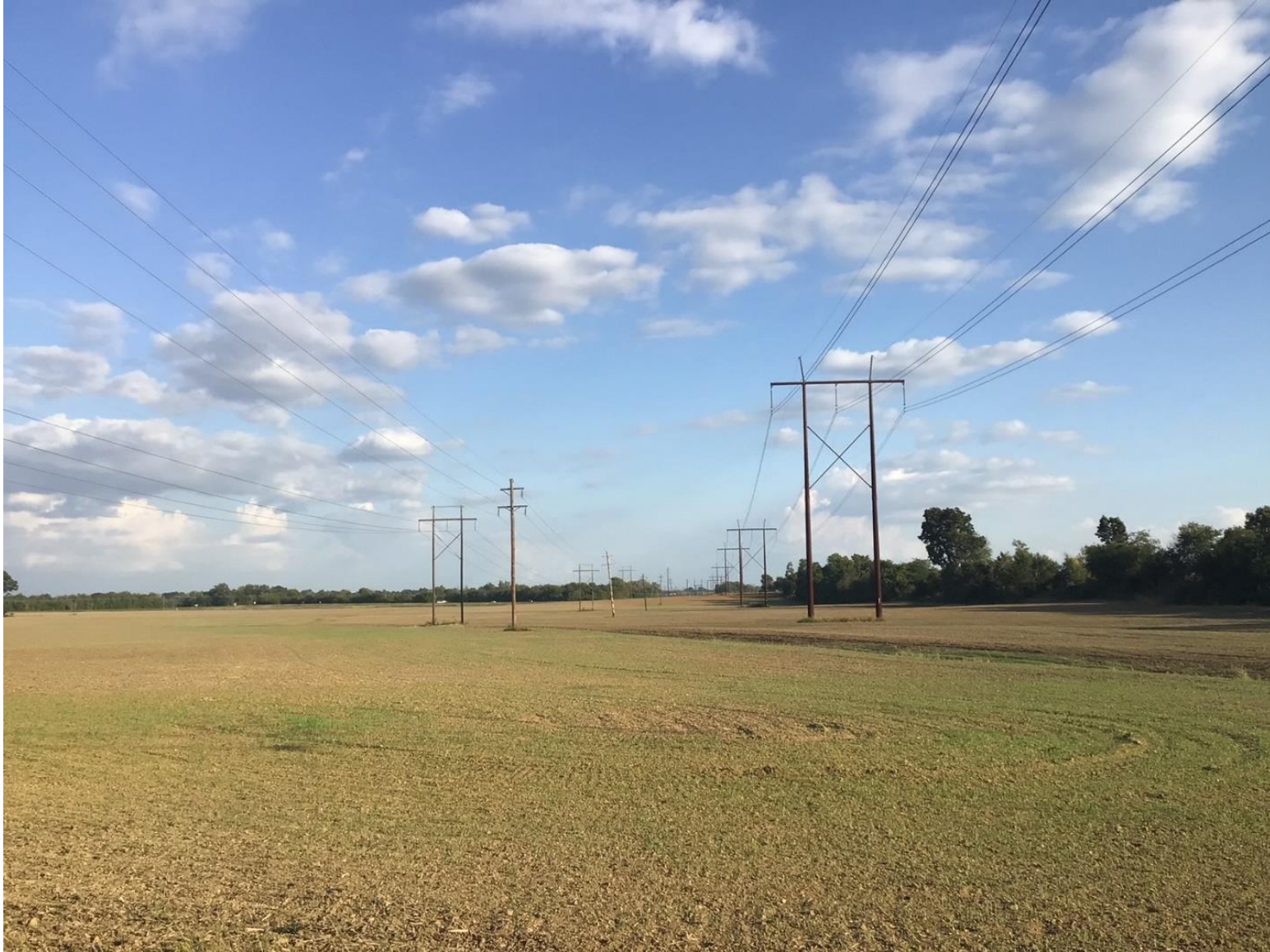
Figure 55 Existing 69 kV, 161 kV, and 345 kV Transmission Lines
