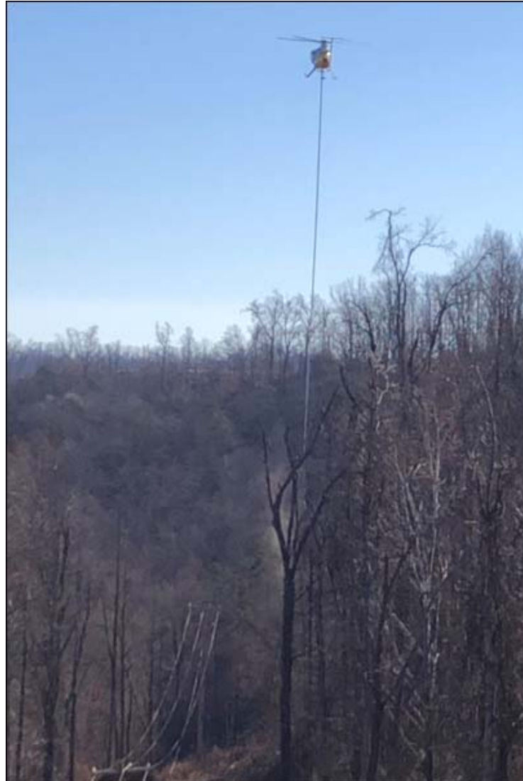
Aerial Saw Work being performed in the Ashland District on the Busseyville Mattie Circuit. This is a remote area adjacent to Yatesville Lake. Picture was taken on December 13, 2021.
