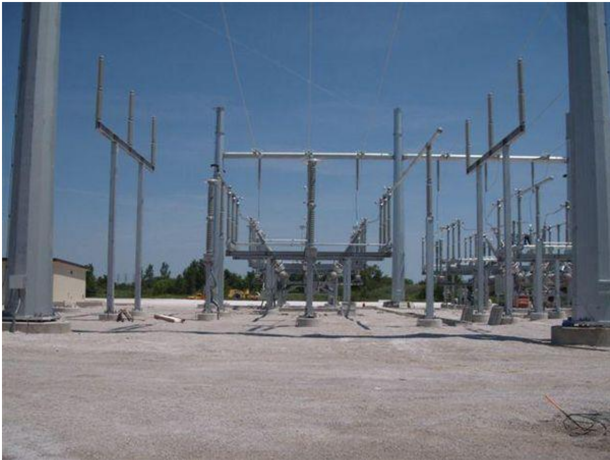
Figure (7) Steel Structures within a Substation 7
