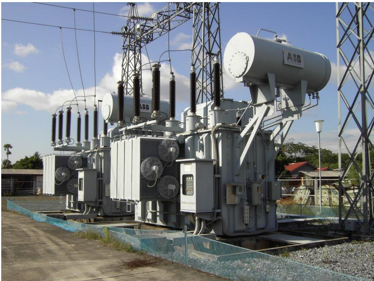
Figure (6) Substation Transformer 6
