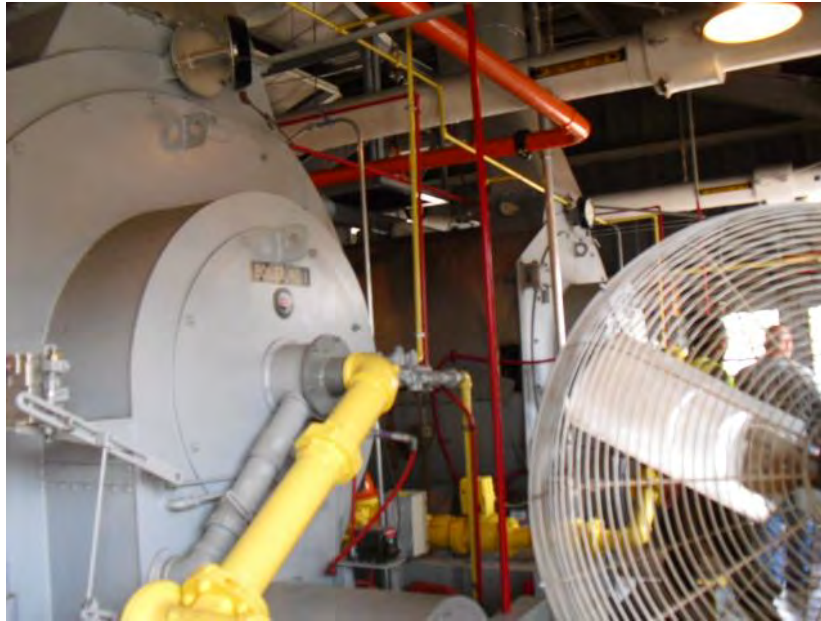
Figure 54: Erlanger Plant Steam Generators
