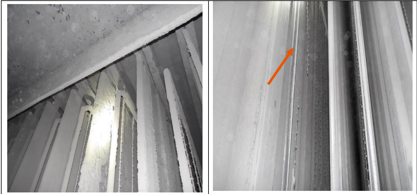
Top Left: A general view of the tops of fields. Top Right and Bottom Left: Examples of broken wires found and removed through out ESP. Bottom Right: Examples of debris found in the ESP from previous outages. This was observed in both Unit 1 and Unit 2.
