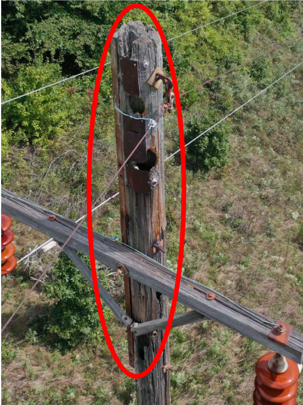
Spring Fork Tap 2 Structure K335-9 Pole rot with temporary braces in place Page 1 of 1
