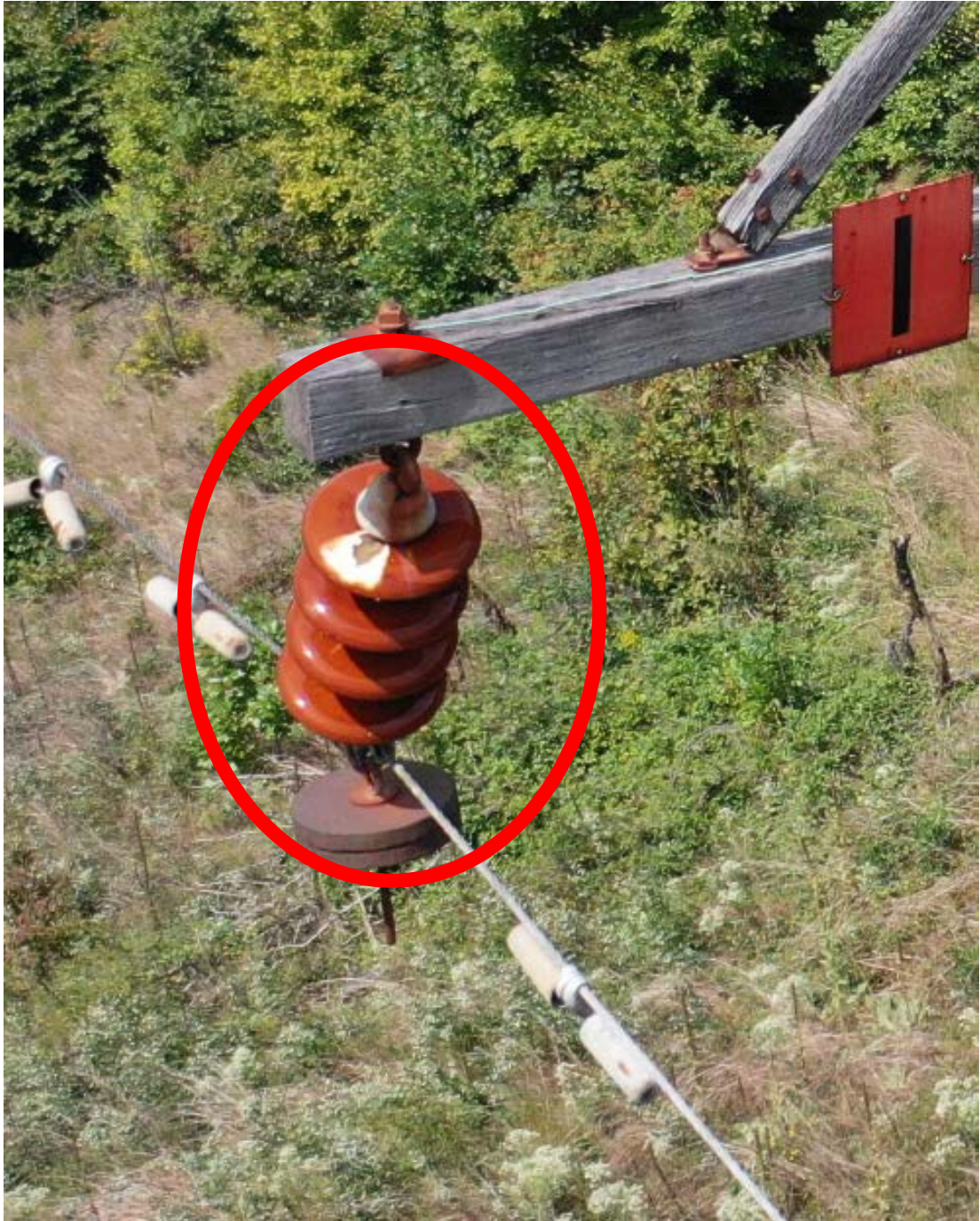
Spring Fork Tap Structure K335-10 Flashover-arcing damage to insulator Page 1 of 1
