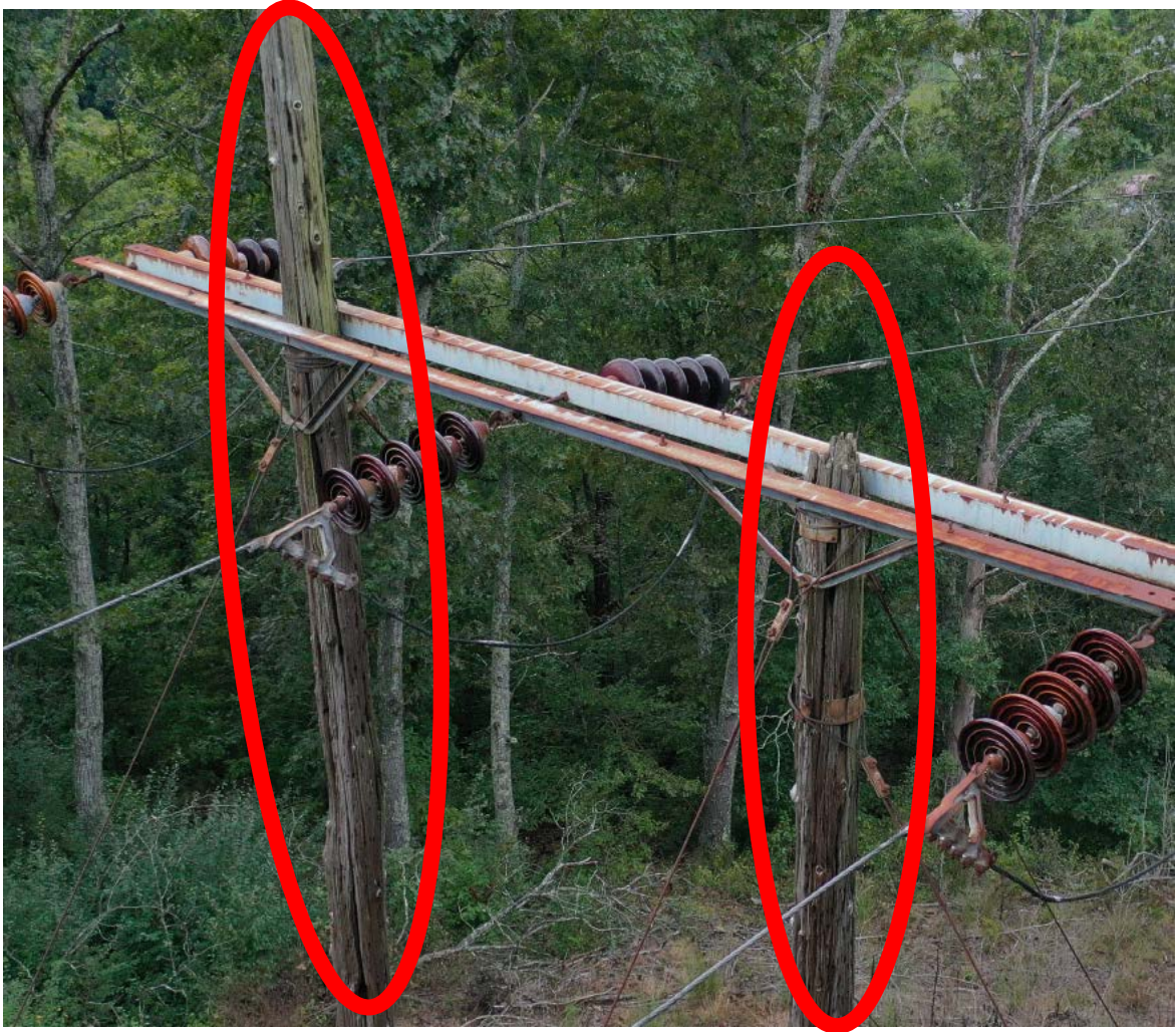
McKinney-Garrett 4 Structure K337-24 Severe Pole Splitting Page 1 of 1
