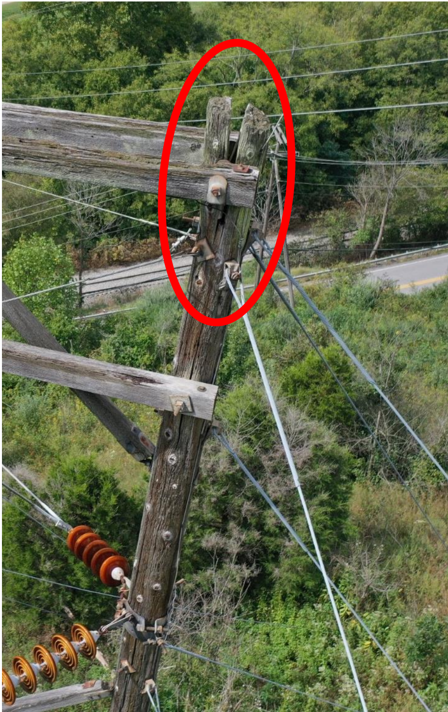
Beaver Creek-Garrett 3 Structure K336-58 Upper pole split to crossarm attachment Page 1 of 1
