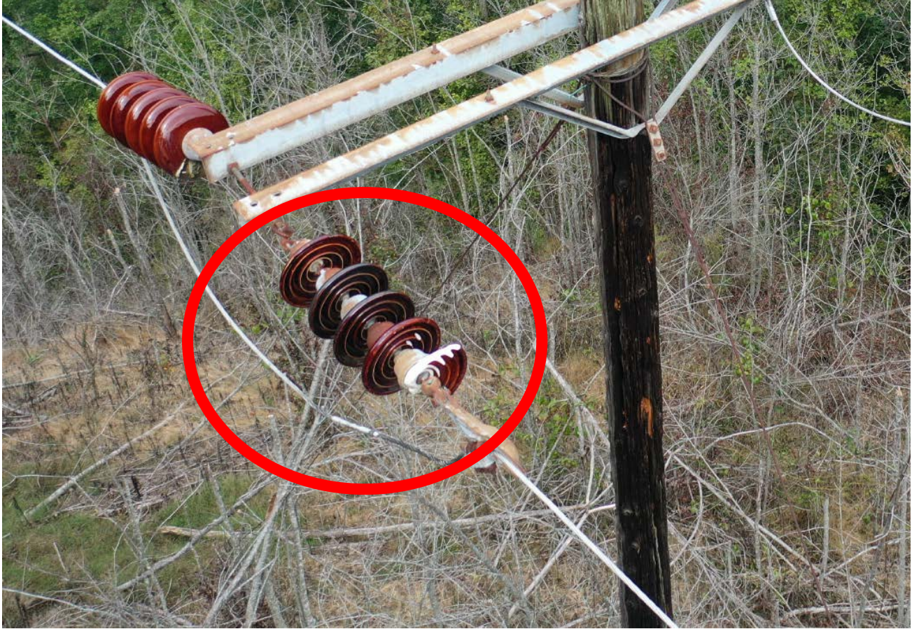
McKinney-Garrett 2 Structure K337-12 One (1) broken insulator in string Page 1 of 1
