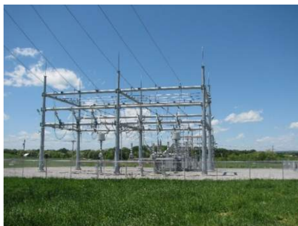
Figure 1: Comparable Proposed Substation
