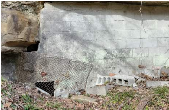
Photograph 3 Gaps in Portal Wall
