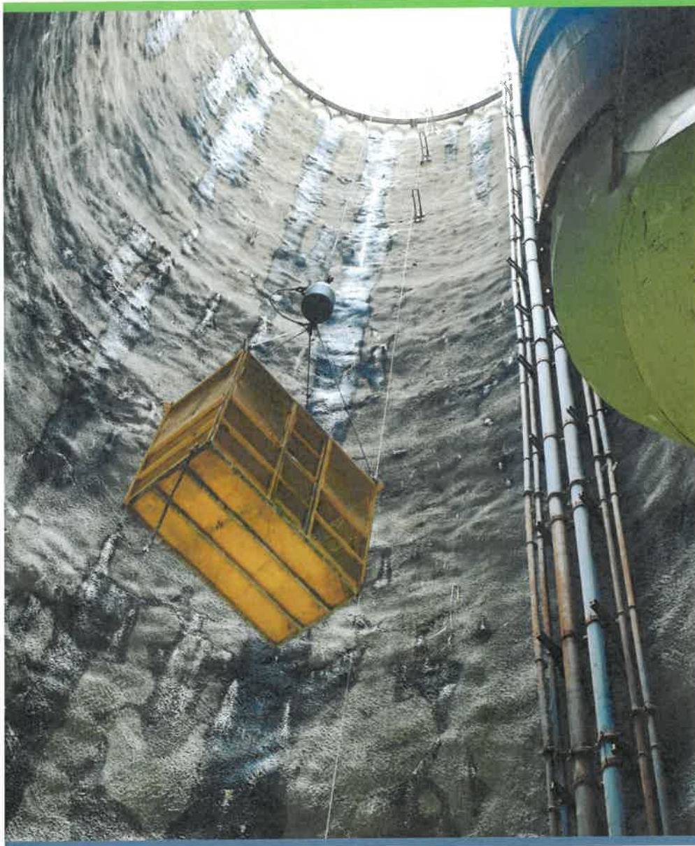
Workers being lowered into MSD's 4-mile Waterway Protection Tunnel. The tunnel will protect the community and our waterways from combined sewer overflows.
