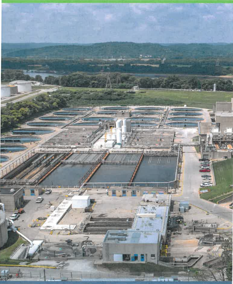
Morris Forman is Kentucky's largest and oldest water quality treatment center. On a normal day, it treats 100 million gallons of wastewater and up to 350 million gallons per day during storms.
